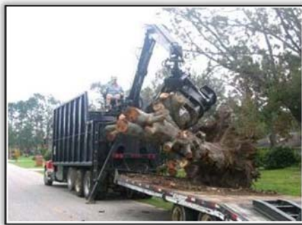
Hazardous Stump Removal
