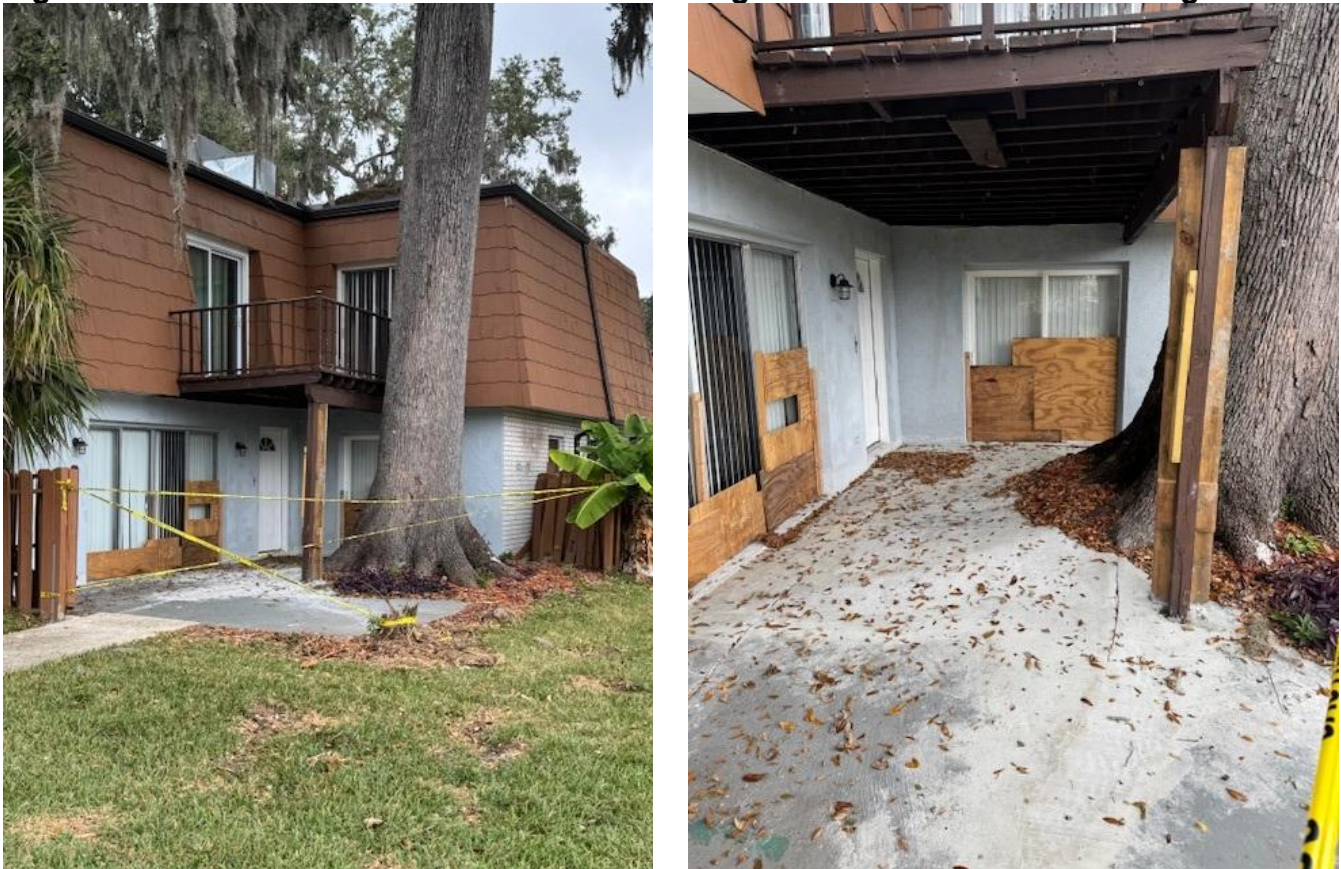
Figure 2. Pictures of the Historic Tree and damage it has caused at 164 Sweetgum Lane
