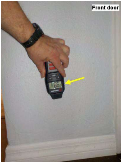
Advise several living room and kitchen walls are 66%-99% wet in numerous areas. Recommend having dehumidifiers placed in unit until moisture intrusion can be controlled.
