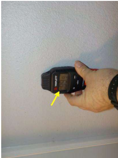
Advise several living room and kitchen walls are 66%-99% wet in numerous areas. Recommend having dehumidifiers placed in unit until moisture intrusion can be controlled.
