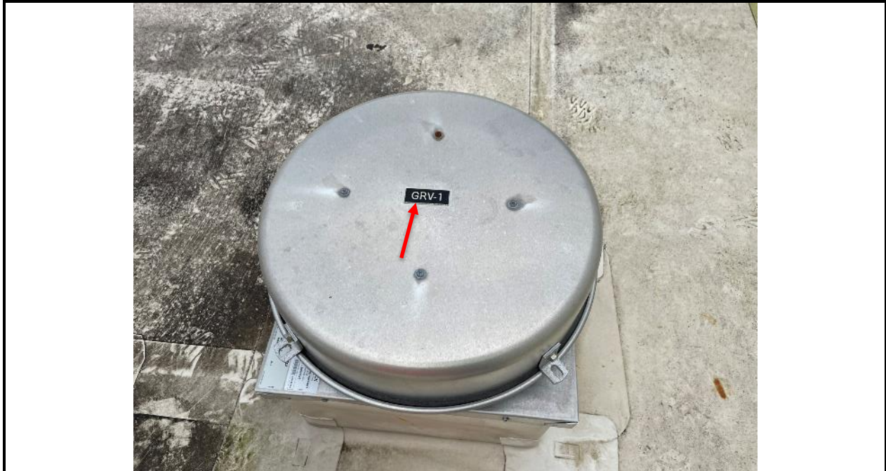
Photo 71: Metal cover at exhaust fan equipment curb (GRV-1) with unsealed fastener penetrations appears to be larger than necessary creating potential avenue for water infiltration.
