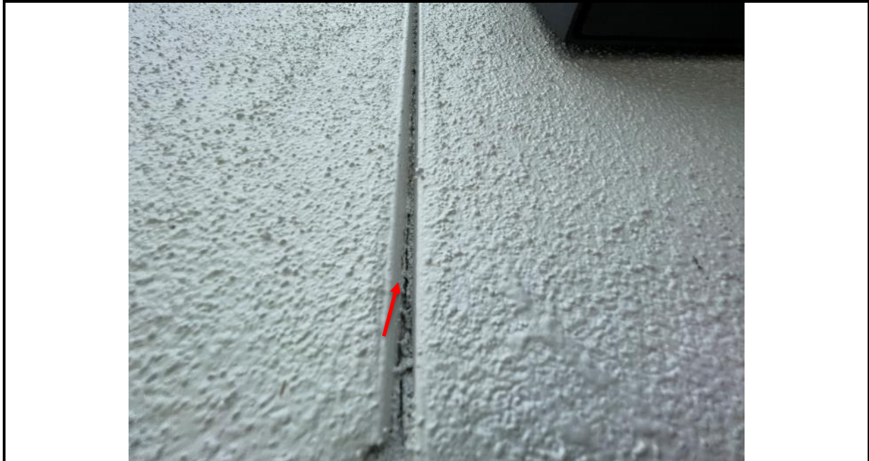
Photo 47: Unsealed transitions at stucco stops.
