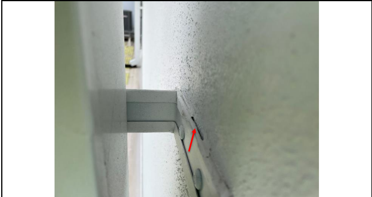
Photo 75: Unsealed brackets at anchoring fasteners associated with downspout systems.
