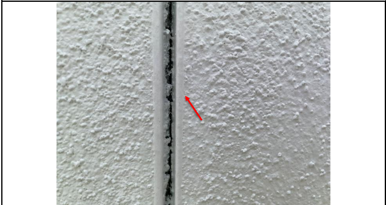
Photo 48: Unsealed transitions at stucco stops.
