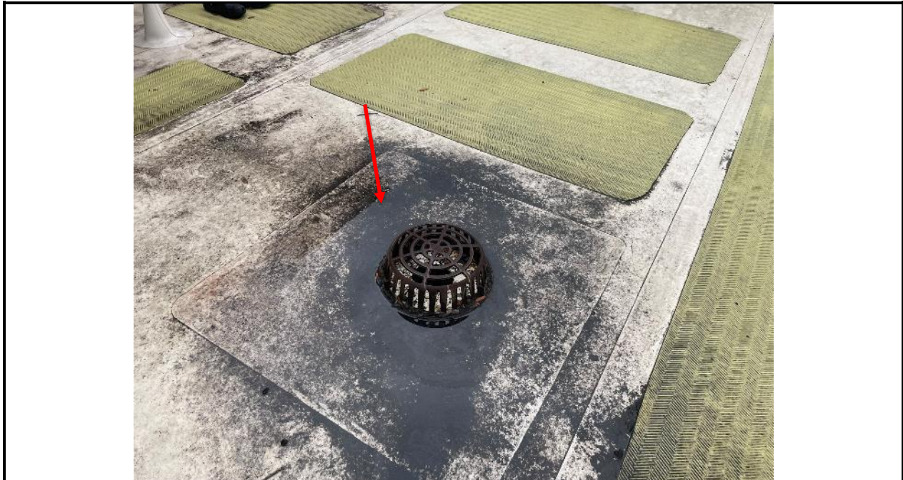
Photo 25: Evidence of current or previously ponded water situated on roofing membrane.
