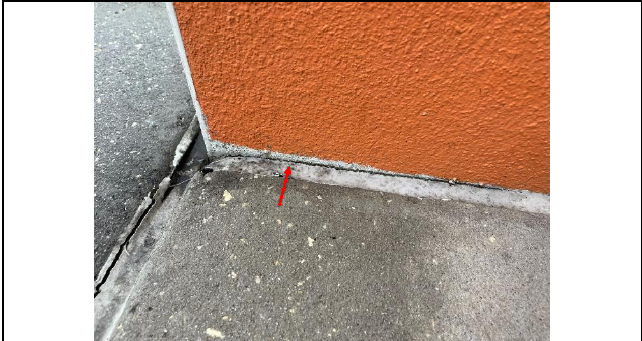
Photo 85: Deteriorated/Missing/Unadhered sealant joint details along concrete flatwork to exterior wall transitions.
