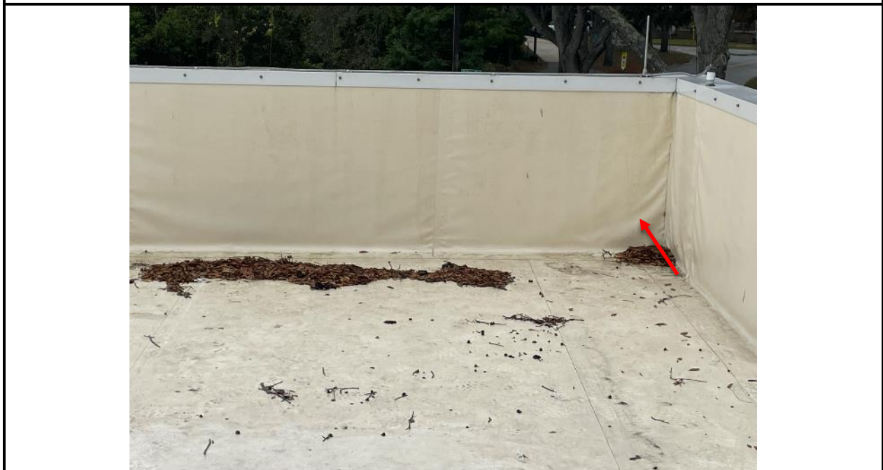
Photo 64: Blisters/Wrinkles in adhered membrane associated with parapet walls.
