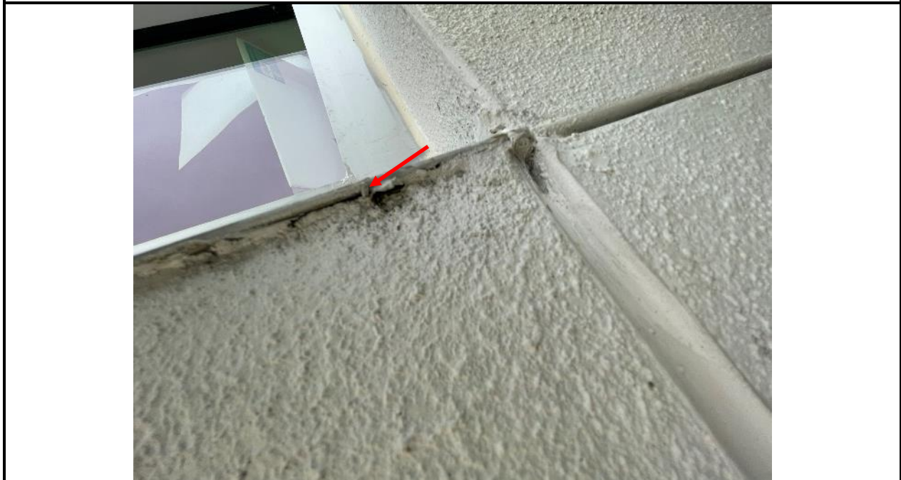
Photo 42: Void beneath windowsill flashings at transition to stucco cladding.
