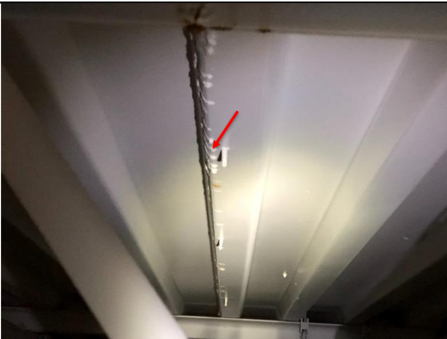
Photo 90: Evidence of previous moisture infiltration including stained interior ceiling components, stained/efflorescence on joists and metal decking, voids in the interior perimeter sealant between window and drywall, and water stains on interior faces of storefront window framing members.
