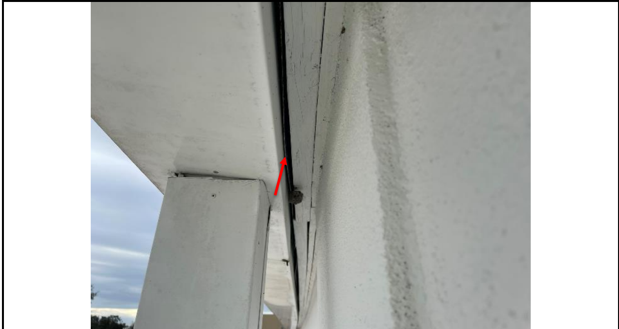
Photo 79: “Fish mouths” appear to be present in the single-ply roofing membrane behind the gutter systems at the wood fascia.
