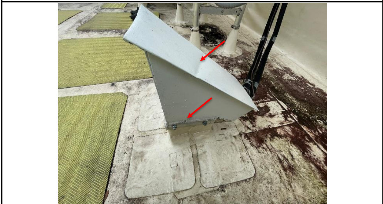
Photo 36: Damaged gooseneck HVAC conduit housing with voids along sealant joints.
