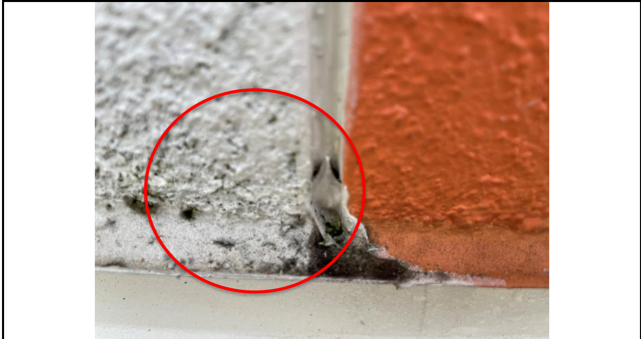
Photo 29: Deteriorated/Missing sealant along joints at building component transitions
