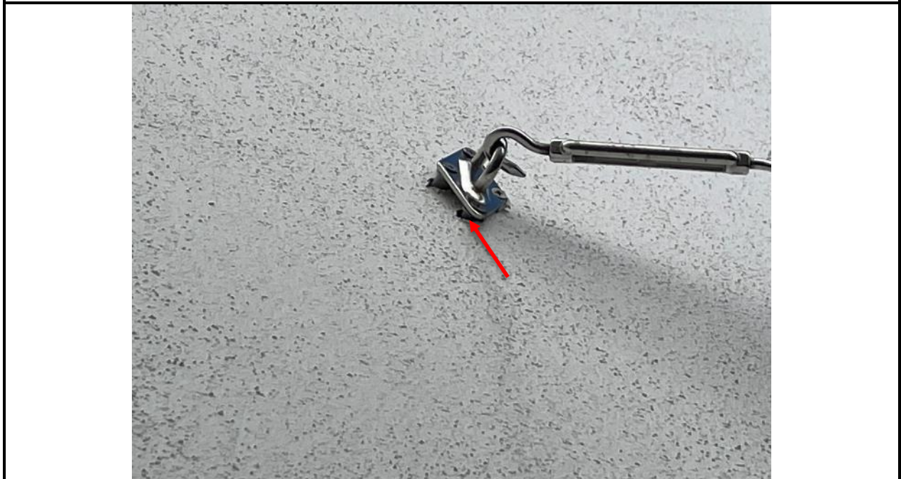
Photo 50: Unsealed through-wall penetrations.
