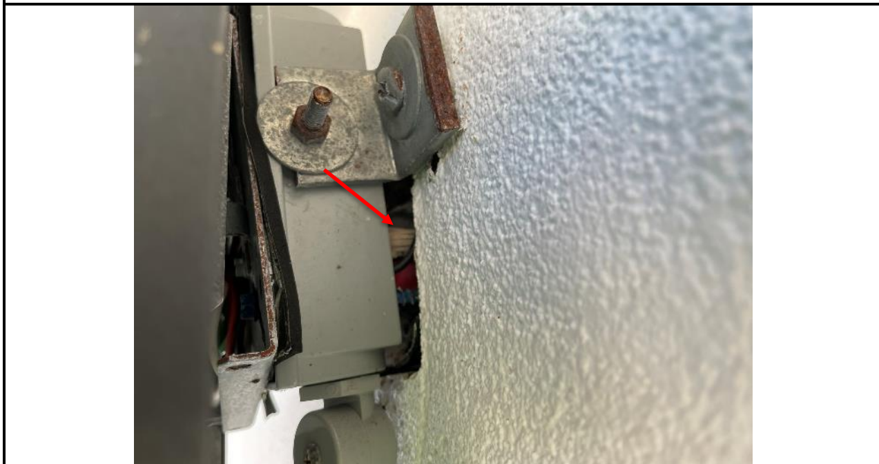
Photo 116: Test location # 5 - NOVA opted not to apply water to the light fixture that appeared unsecured and unsealed to exterior wall systems exposing electrical wiring behind the exterior cladding due to safety reasons.
