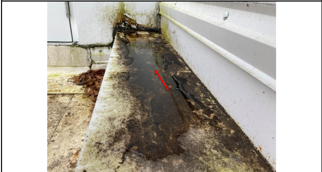
Photo 66: Metal coping cap appears to consist of negative slopes and retaining water creating stains and mildew growth.
