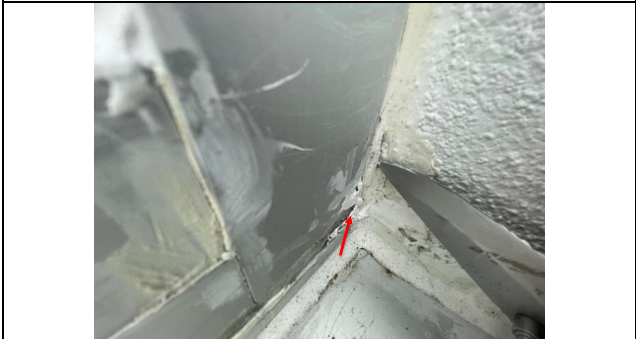
Photo 44: Void in sealant along window perimeter sealant joint transition to adjacent construction.
