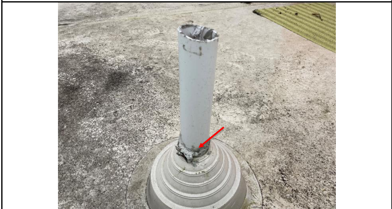
Photo 38: Deteriorated/Missing sealant at roof penetration transitions.
