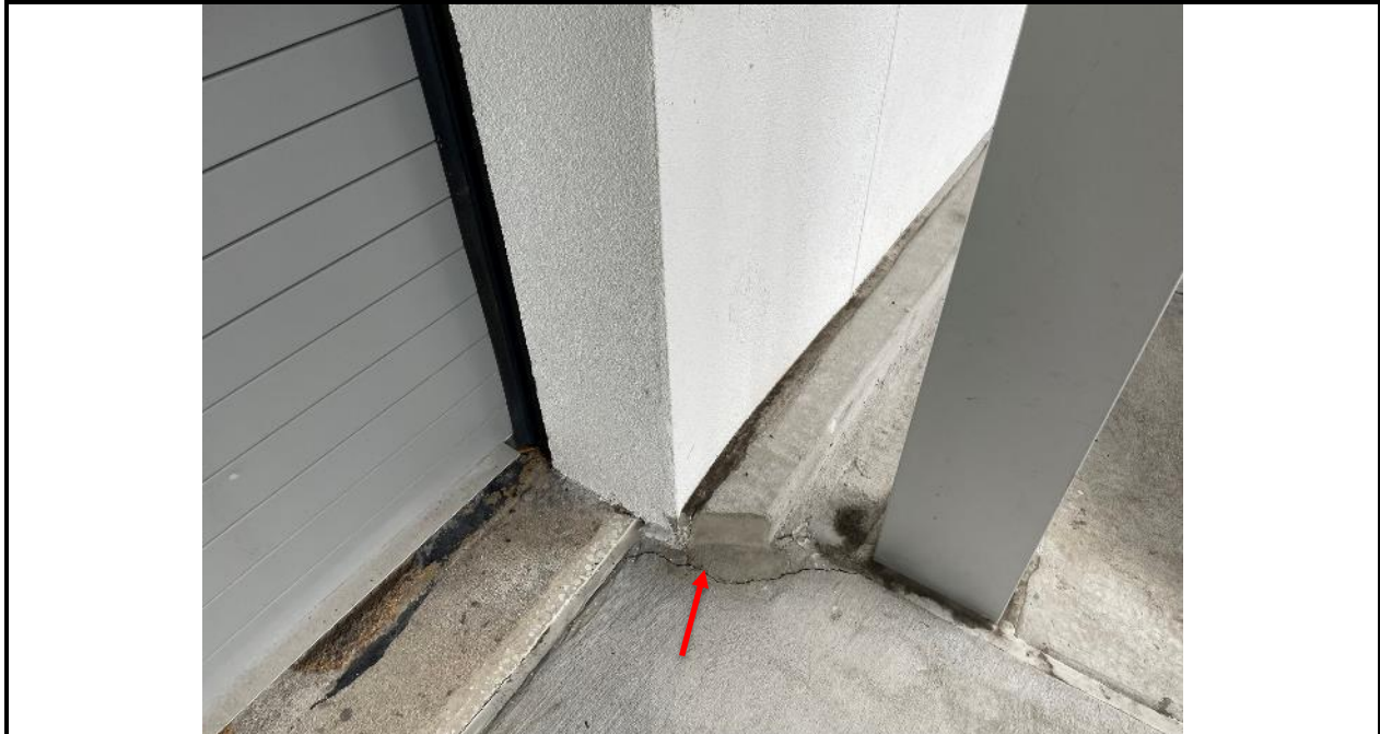
Photo 87: Crack formations throughout concrete flatwork.
