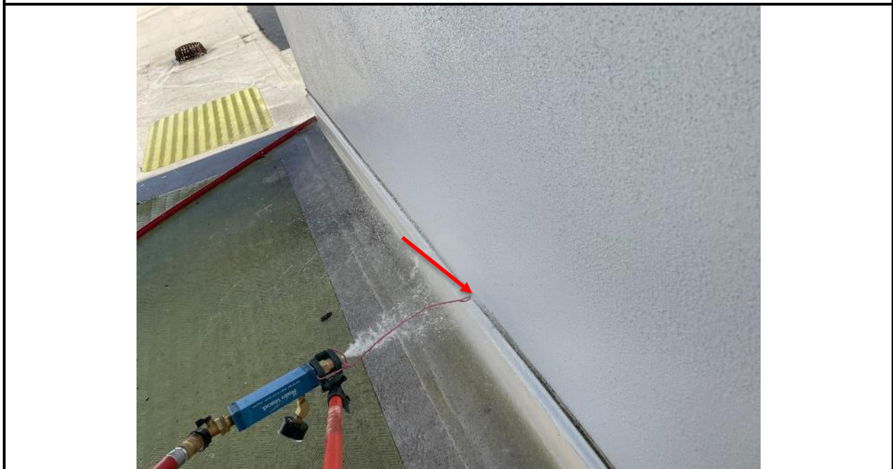
Photo 104: Test location #1 - water was applied along the metal counter flashing transitions with voids in the sealant joints between the 1 st floor roof membrane and the adjacent construction (stair tower).
