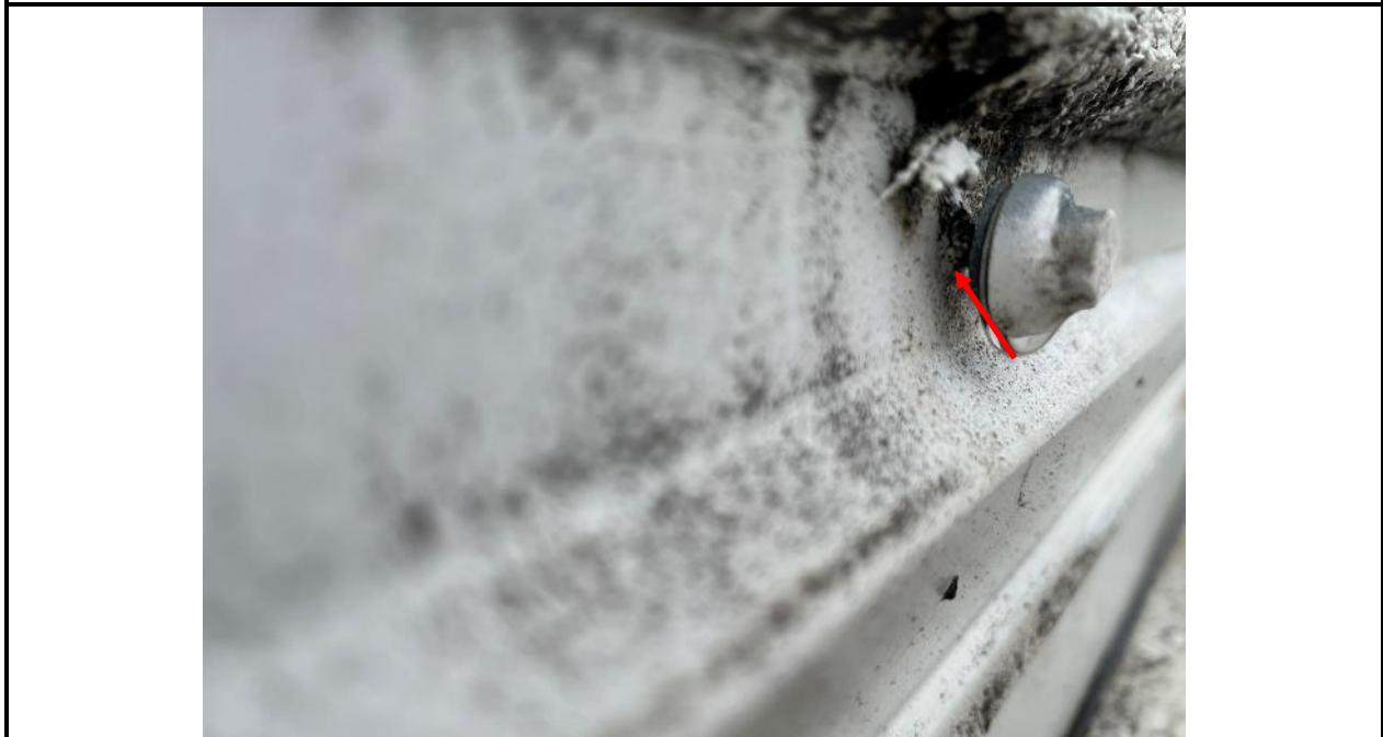
Photo 78: Withdrawn fasteners with neoprene washers associated with roof metal counter flashing at transition to adjacent construction.
