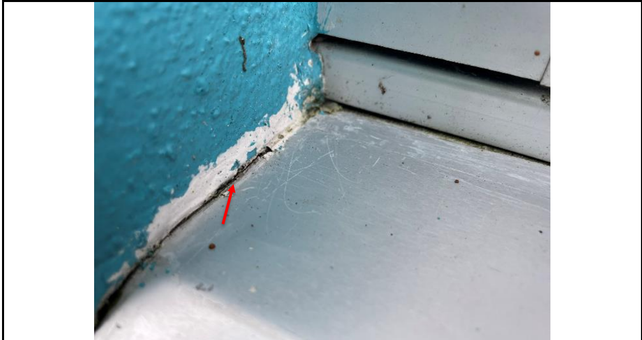
Photo 61: Openings at window assemblies' sill flashing corner transitions to adjacent construction.
