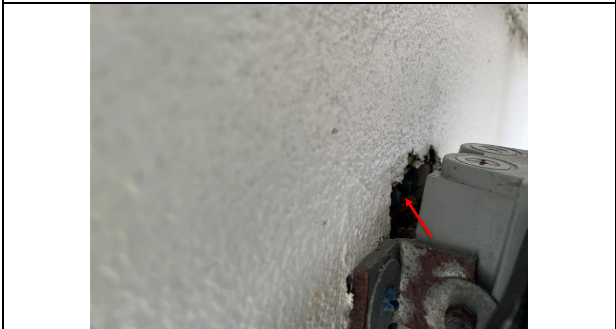
Photo 80: Light fixtures unsecured and unsealed to exterior wall systems exposing electrical wiring behind.
