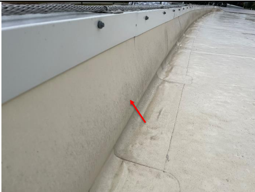
Photo 82: Unadhered single-ply roofing membrane along parapet walls.
