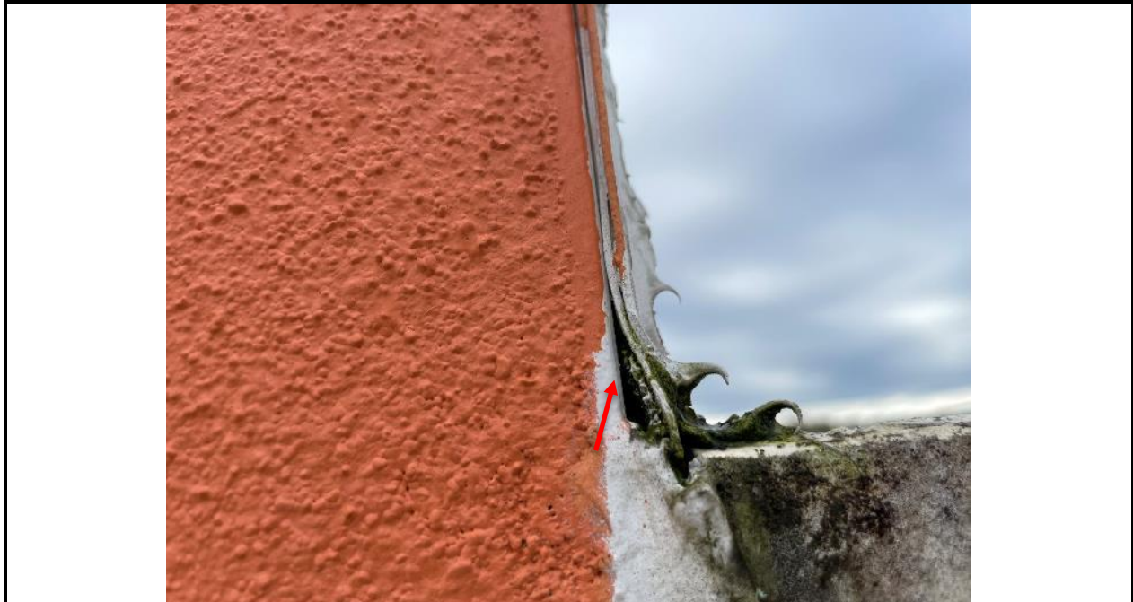
Photo 69: Separation at roof membrane transition to stucco cladding associated with elevator penthouse.
