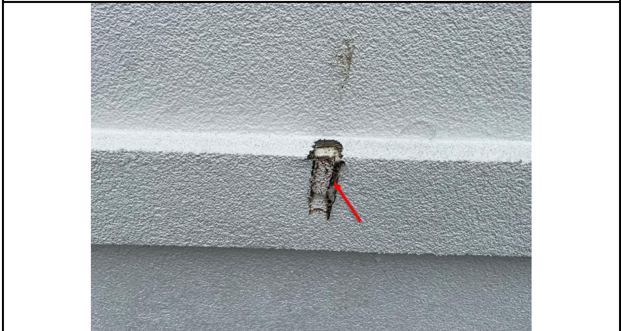
Photo 58: Damaged exterior cladding.
