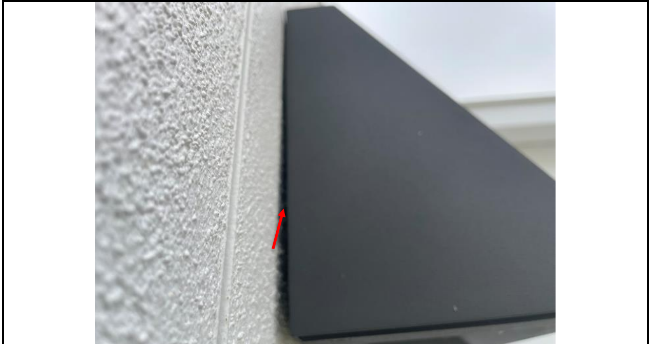
Photo 51: Unsealed through-wall penetrations.
