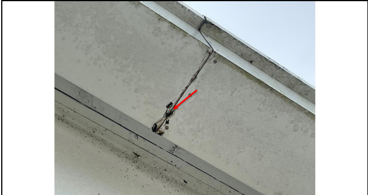
Photo 35: Damaged gutter systems create dripping conditions onto roof systems below.
