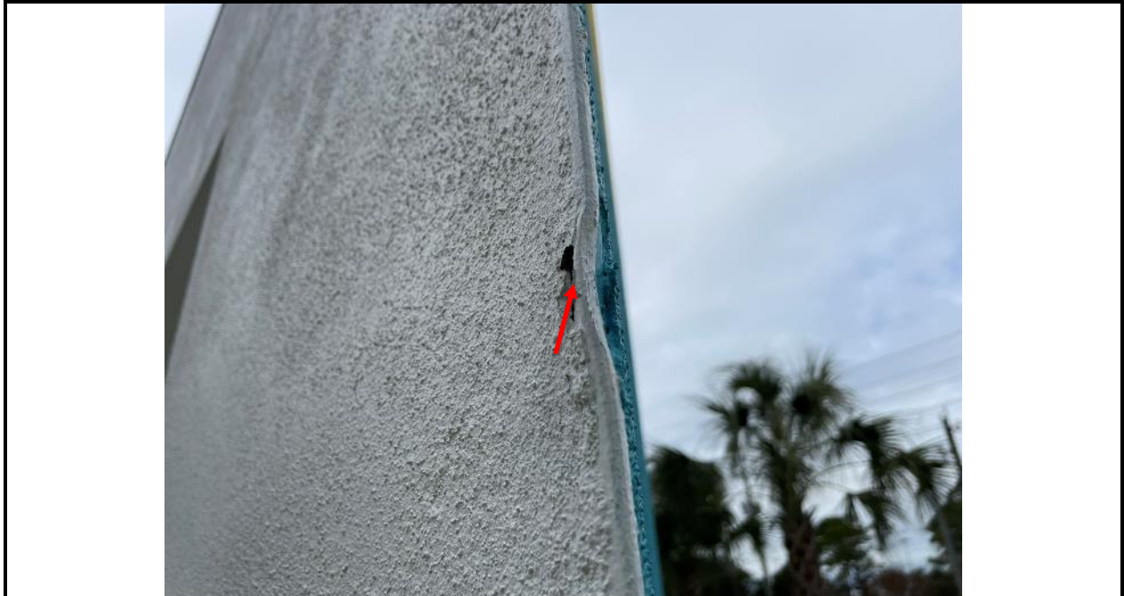
Photo 57: Damaged exterior cladding.
