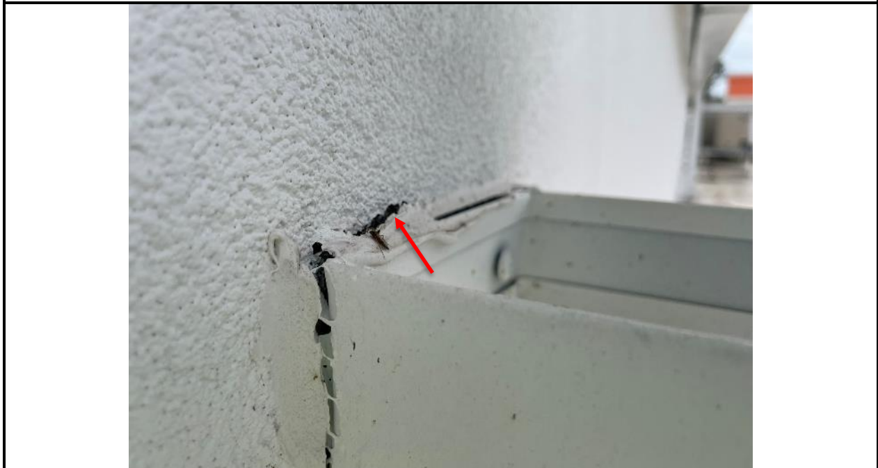
Photo 76: Unsealed brackets at anchoring fasteners associated with downspout systems.
