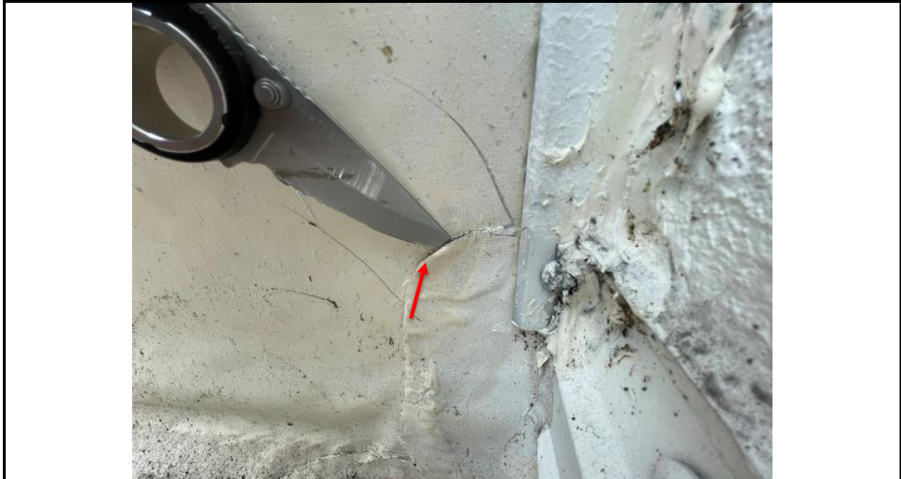
Photo 63: Unadhered membrane patch along parapet walls.
