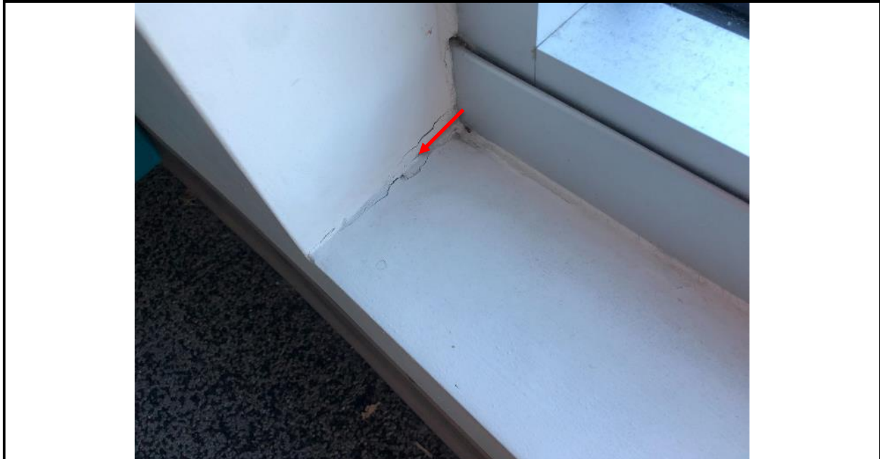
Photo 93: Evidence of previous moisture infiltration including stained interior ceiling components, stained/efflorescence on joists and metal decking, voids in the interior perimeter sealant between window and drywall, and water stains on interior faces of storefront window framing members.
