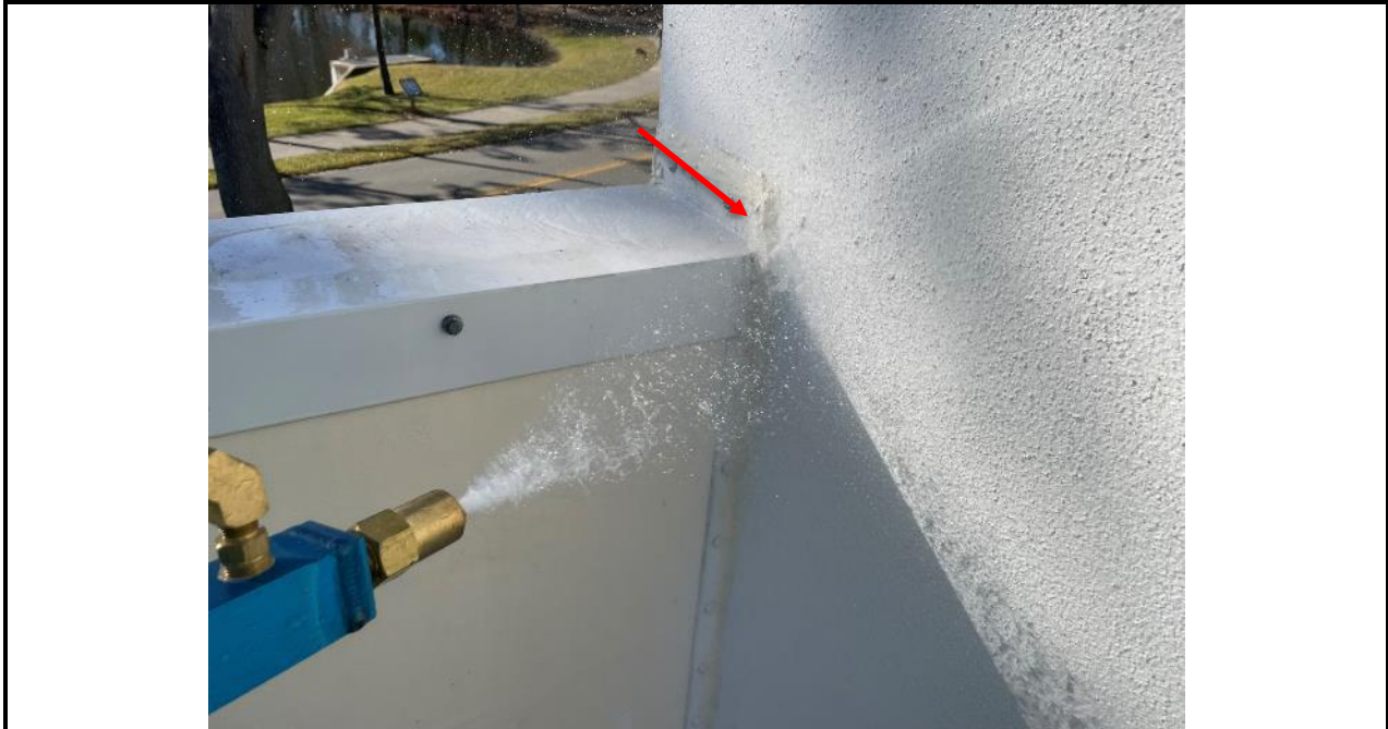
Photo 119: Test location # 6 - water was applied along the voids in the vertical and horizontal sealant joints at the parapet wall transition to adjacent construction, and the observed unadhered membrane patch at the parapet wall corner.
