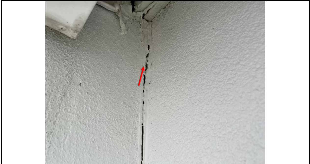
Photo 67: Cohesive failure at sealant joint detail between original and addition construction.
