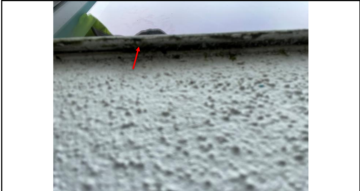
Photo 43: Void beneath windowsill flashings at transition to stucco cladding.
