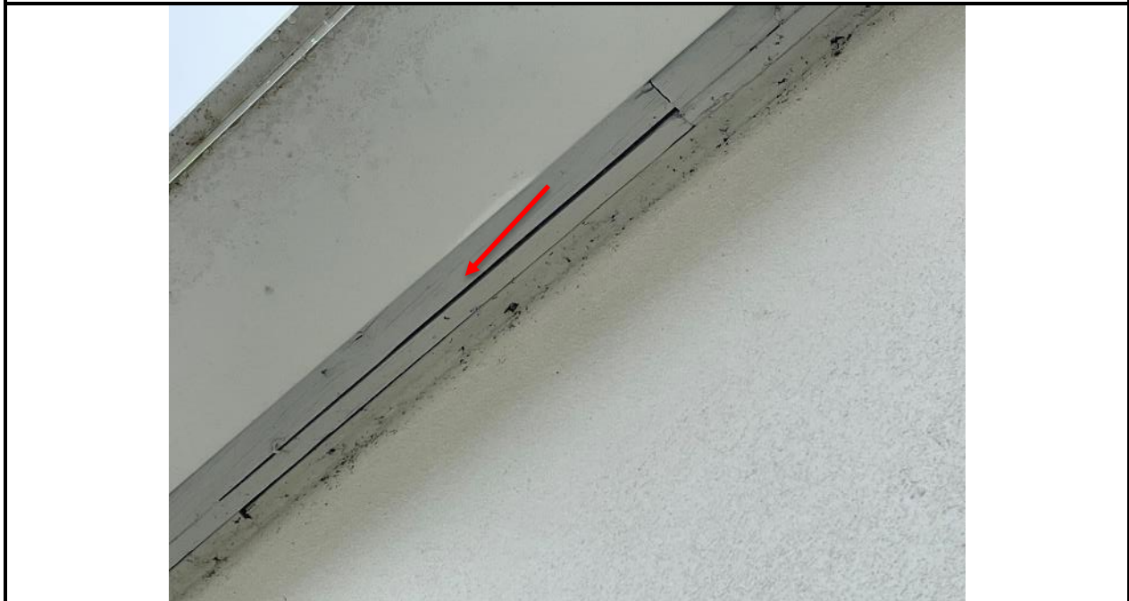
Photo 34: Spacing without sealant joint associated with wood fascia behind gutter systems.
