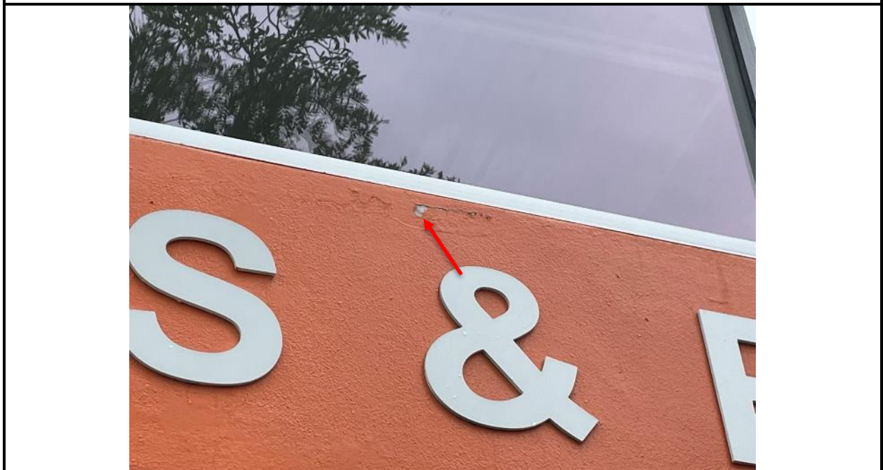
Photo 84: Blistered/Peeled paint finishes throughout stucco cladding.
