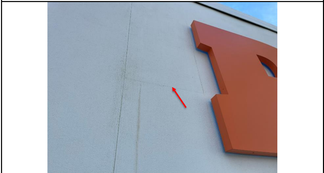
Photo 54: Crack formations associated with exterior façades.
