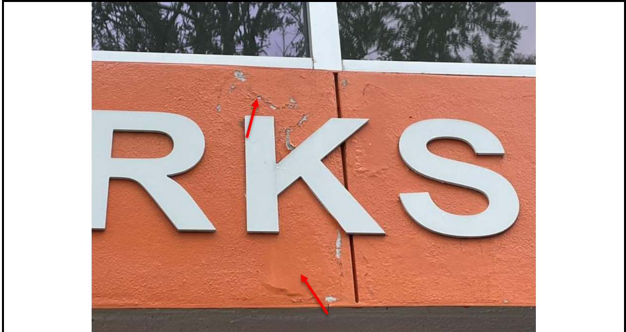
Photo 83: Blistered/Peeled paint finishes throughout stucco cladding.
