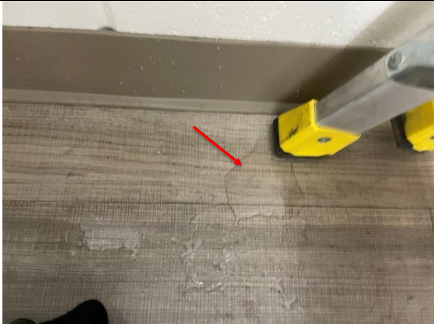
Photo 113: Test location #3 - water was visually observed ponding on the internal threshold of the access door and cascading down the interior face of the gypsum wallboard eventually collecting on the finished flooring within minutes of commencing testing.
