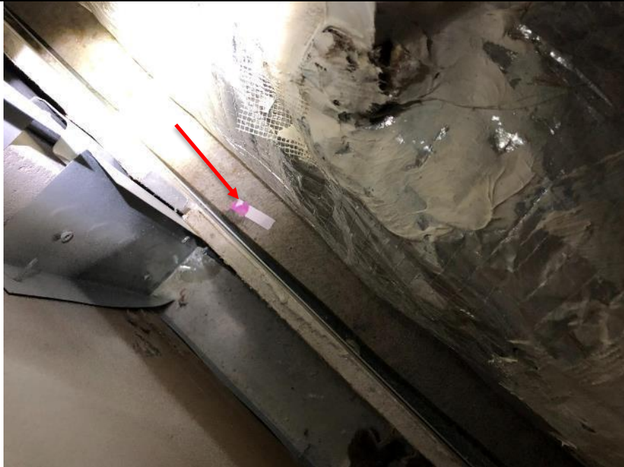
Photo 109: Test location #2 - water was visually observed and detected utilizing infrared thermography streaming down the CMU block wall at the steel girder/joist and roof deck transition as well as dripping onto the HVAC ductwork and ceiling components.
