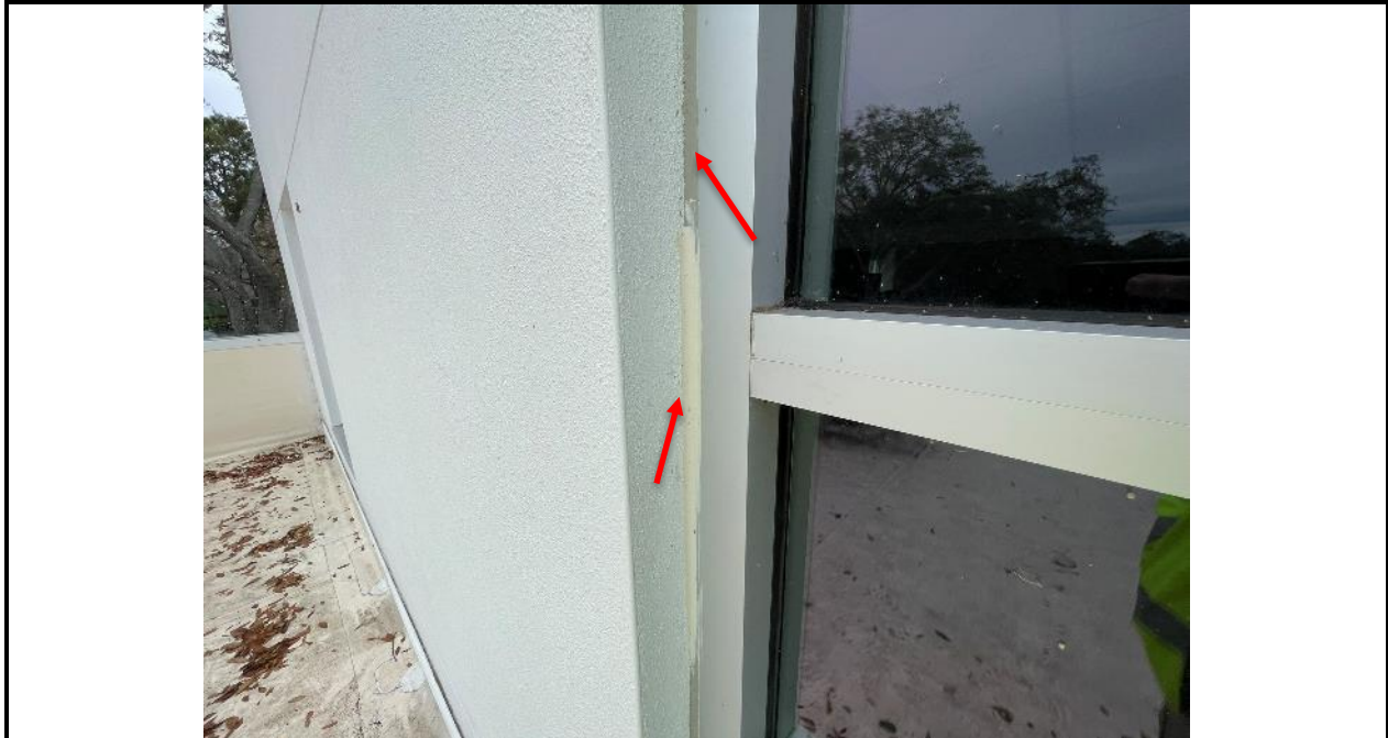
Photo 59: Window perimeter sealant remediations appear incomplete.
