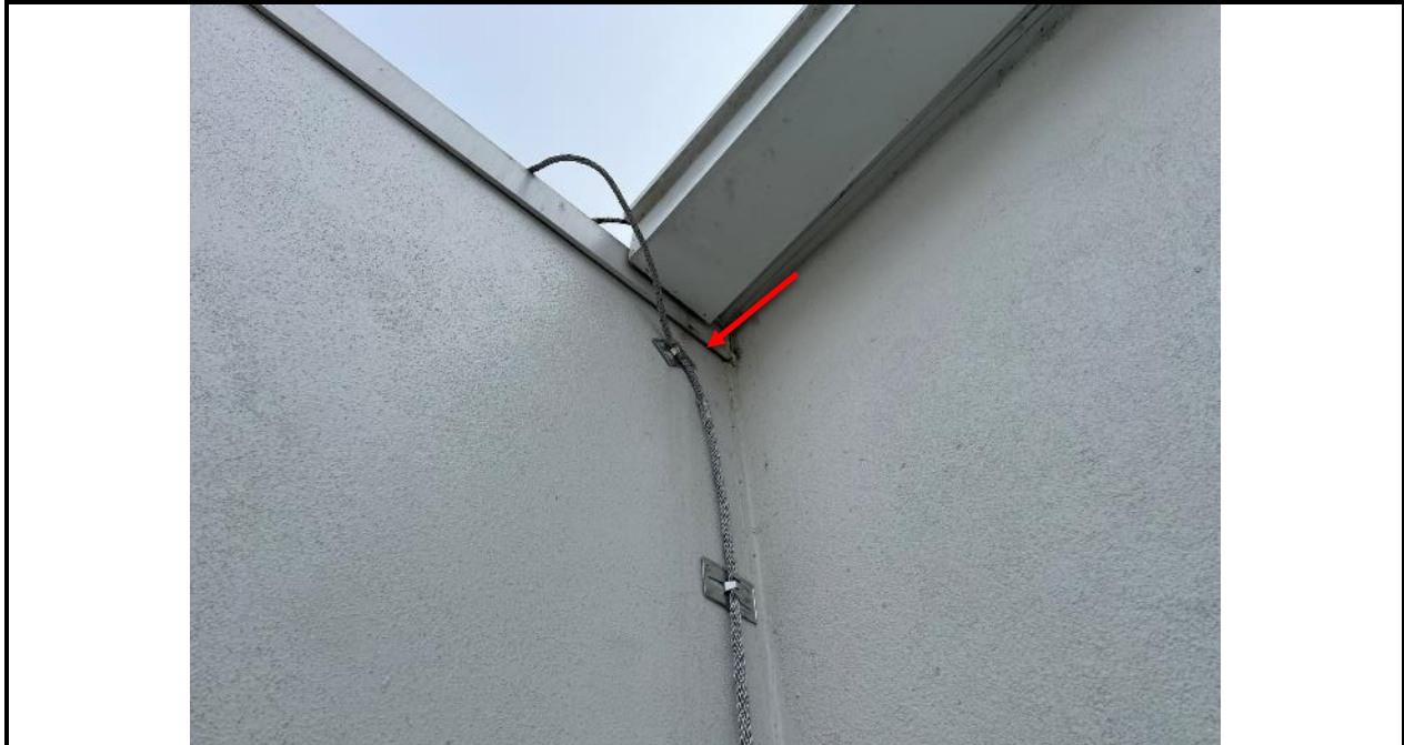
Photo 39: Opening in exterior cladding behind metal drip edge flashing/coping cap associated with roof system.
