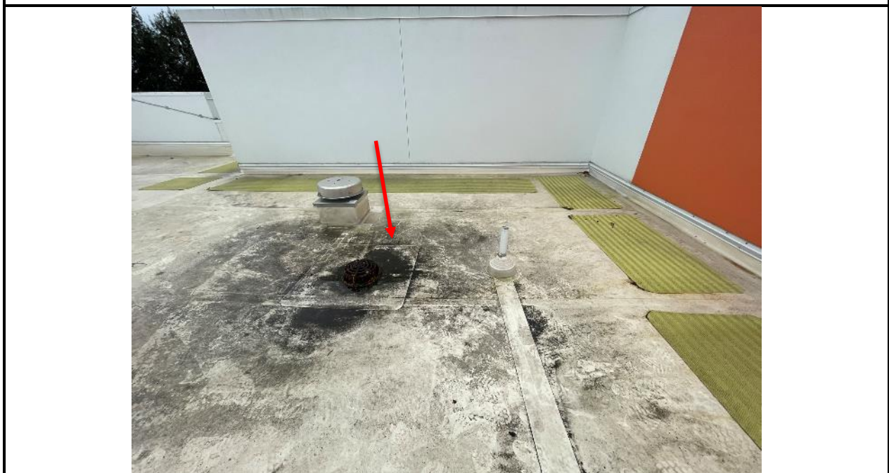
Photo 26: Evidence of current or previously ponded water situated on roofing membrane.
