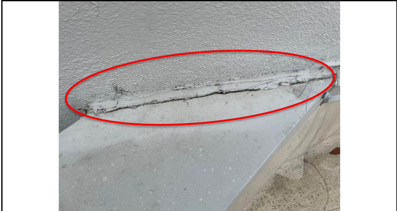
Photo 31: Deteriorated/Missing sealant along joints at building component transitions
