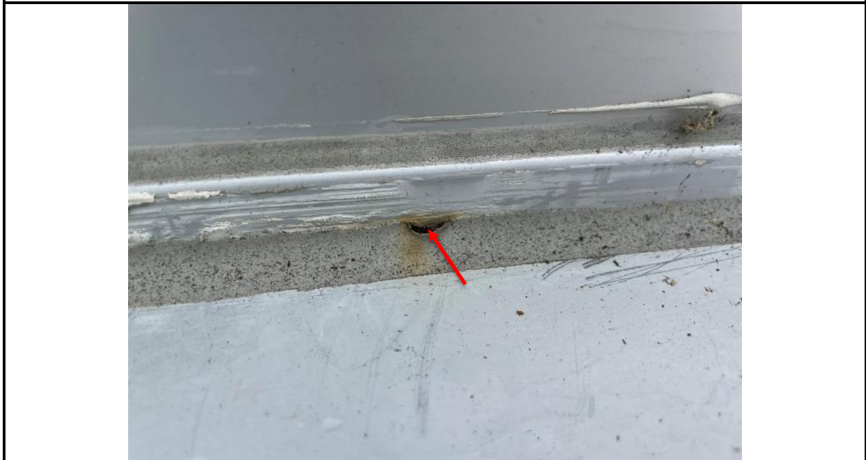
Photo 46: Void in sealant along window perimeter sealant joint transition to adjacent construction.
