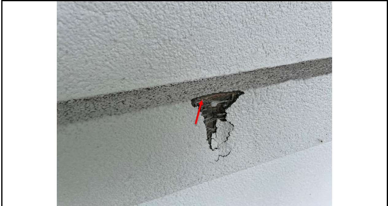
Photo 55: Damaged exterior cladding.
