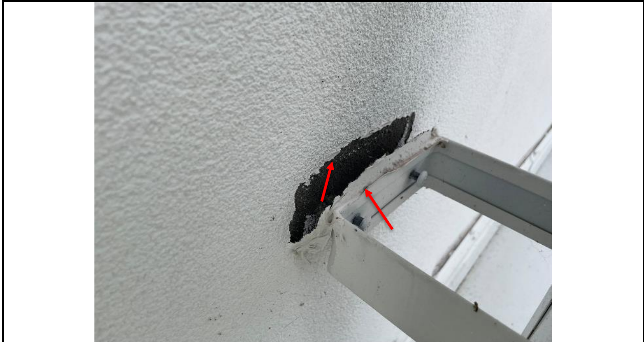
Photo 77: Unsecured anchor fasteners associated with downspout systems.
