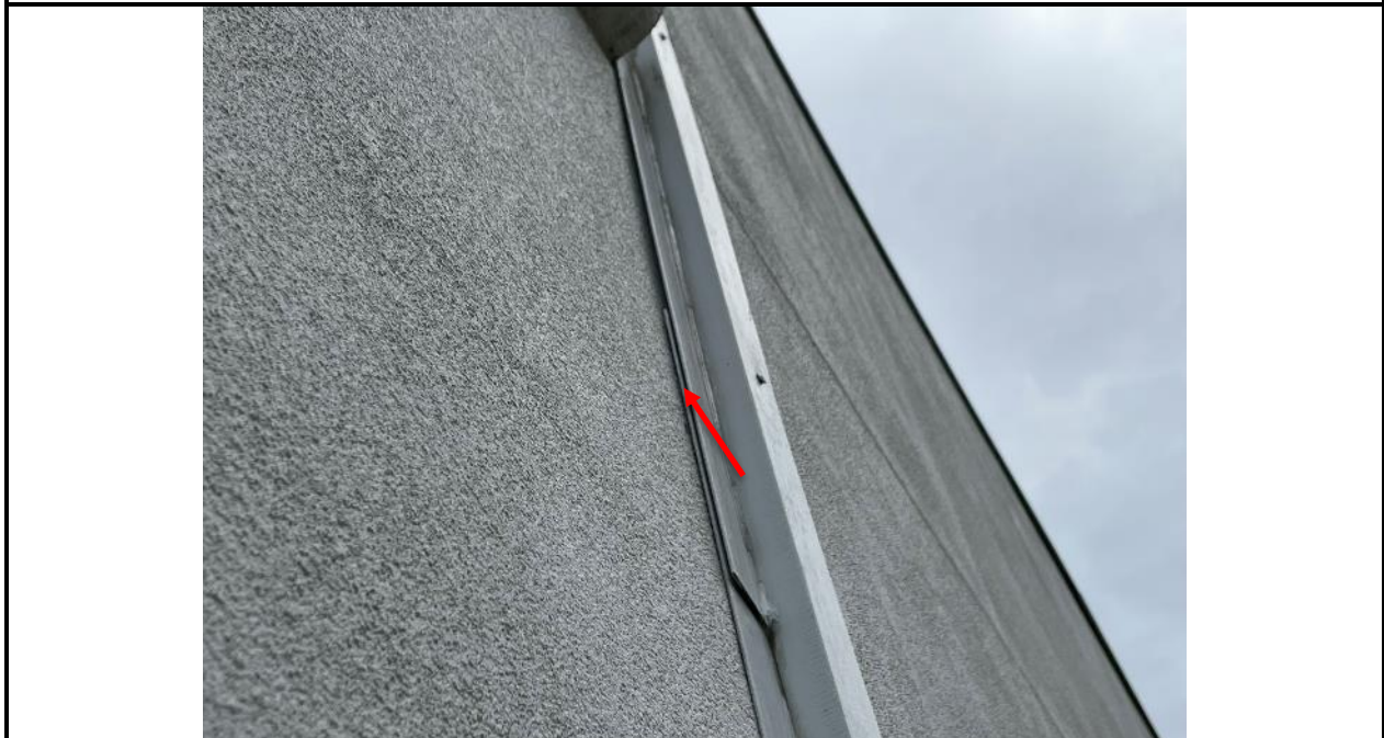
Photo 88: Unsealed transition at metal flashing from original to addition construction.
