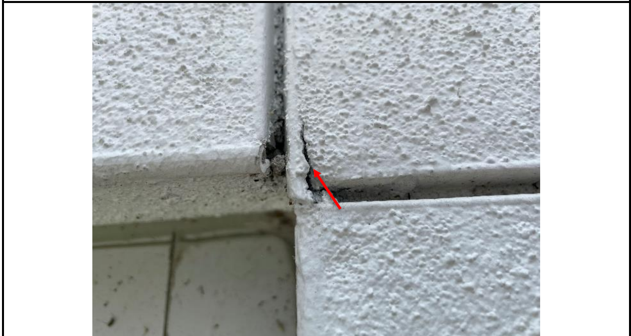
Photo 52: Crack formations associated with exterior façades.
