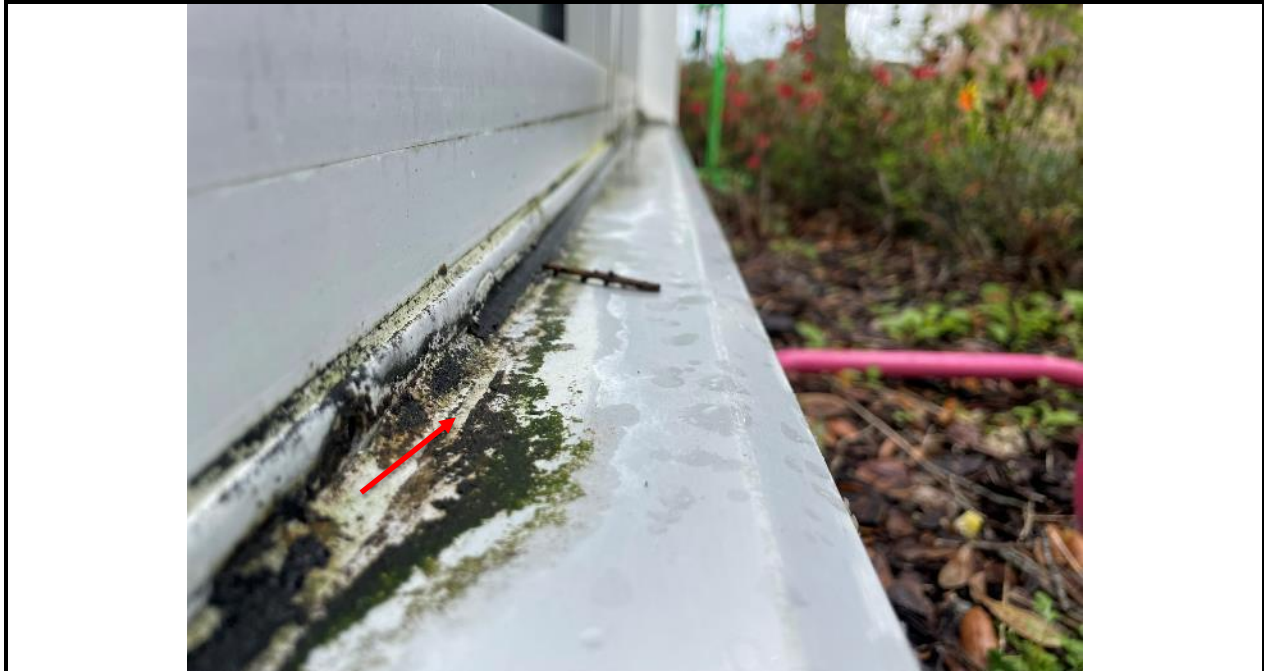
Photo 41: Sill flashing associated with window systems appears to have a negative slope back towards building exteriors creating stains and mildew growth.
