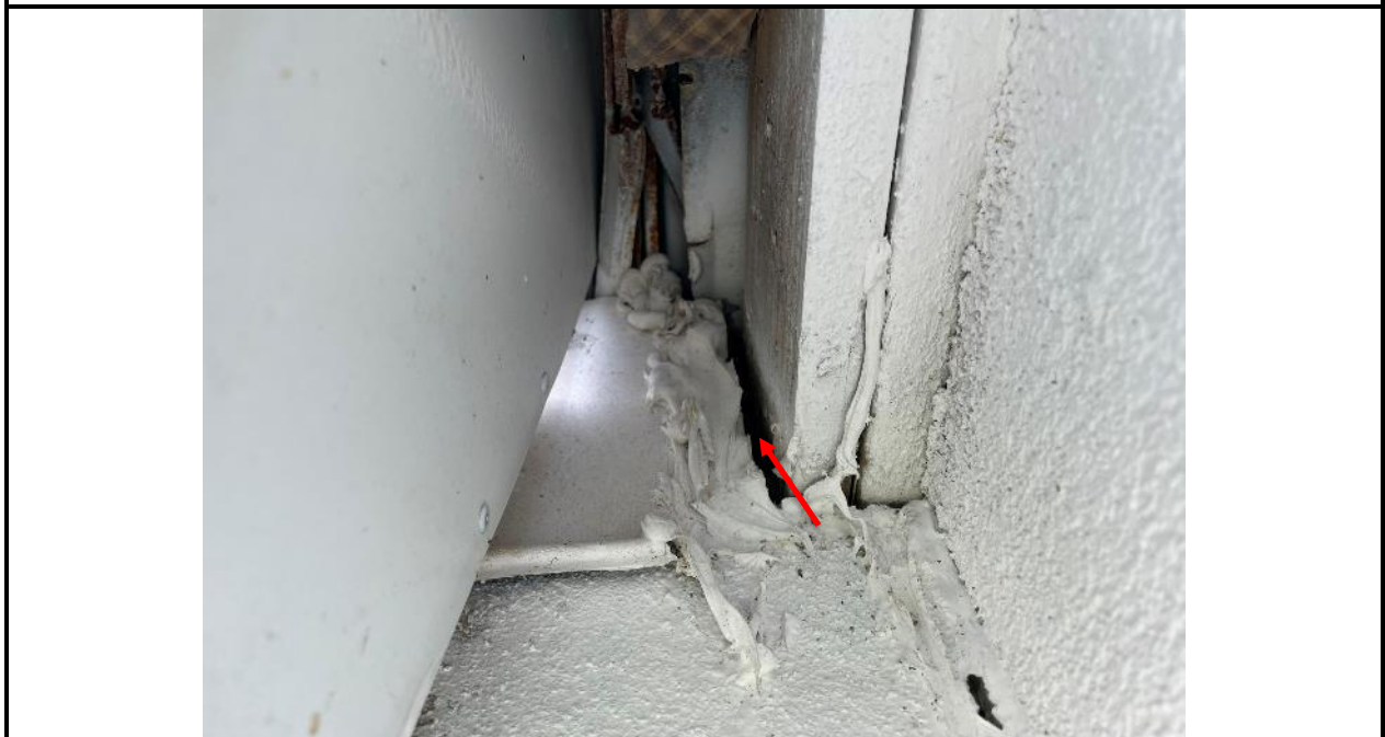
Photo 68: Opening at original to addition construction behind gutter system at wood fascia transition.
