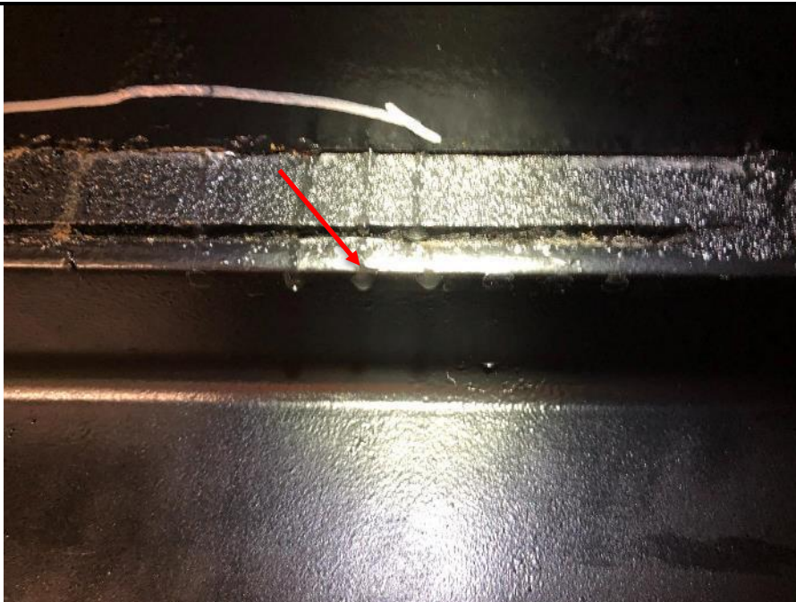
Photo 122: Test location #6 - Water intrusion was observed emanating between the metal roof decking and the steel support framing members eventually dripping onto the furniture below when testing both sill conditions.
