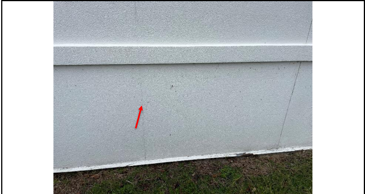
Photo 53: Crack formations associated with exterior façades.
