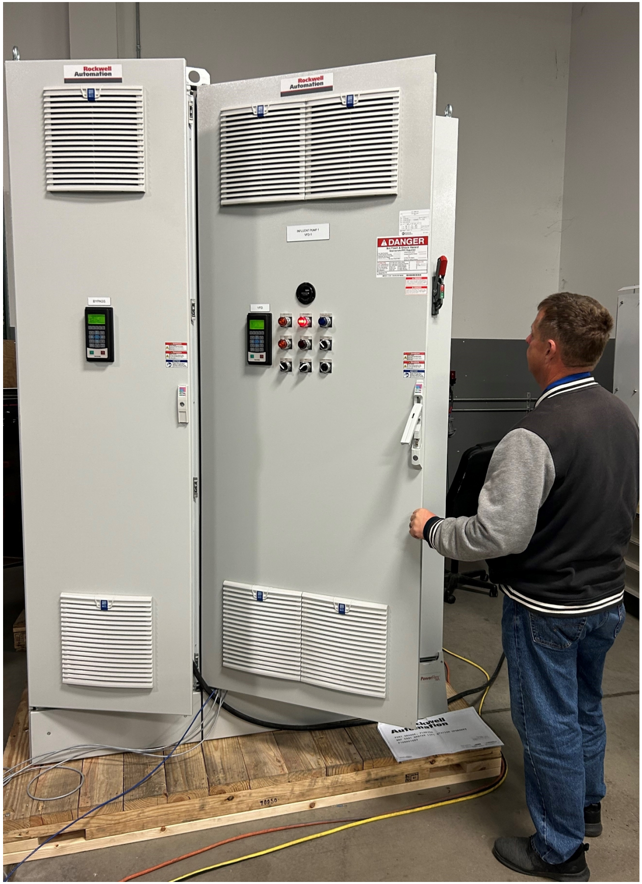
City Staff Inspecting a Variable Frequency Drive (VFD) for Witness Testing
