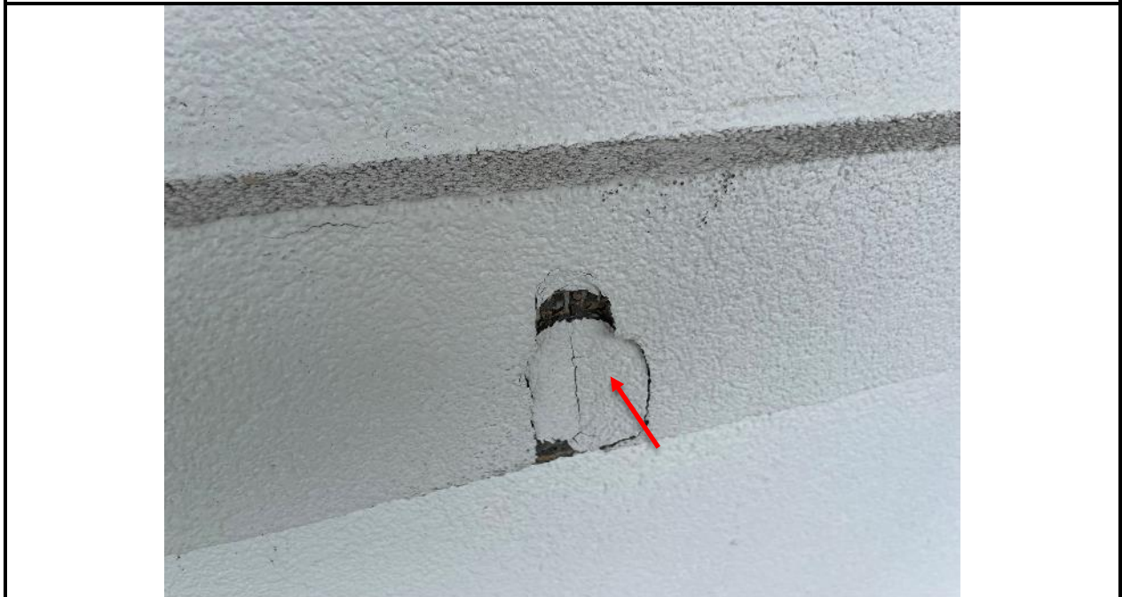
Photo 56: Damaged exterior cladding.
