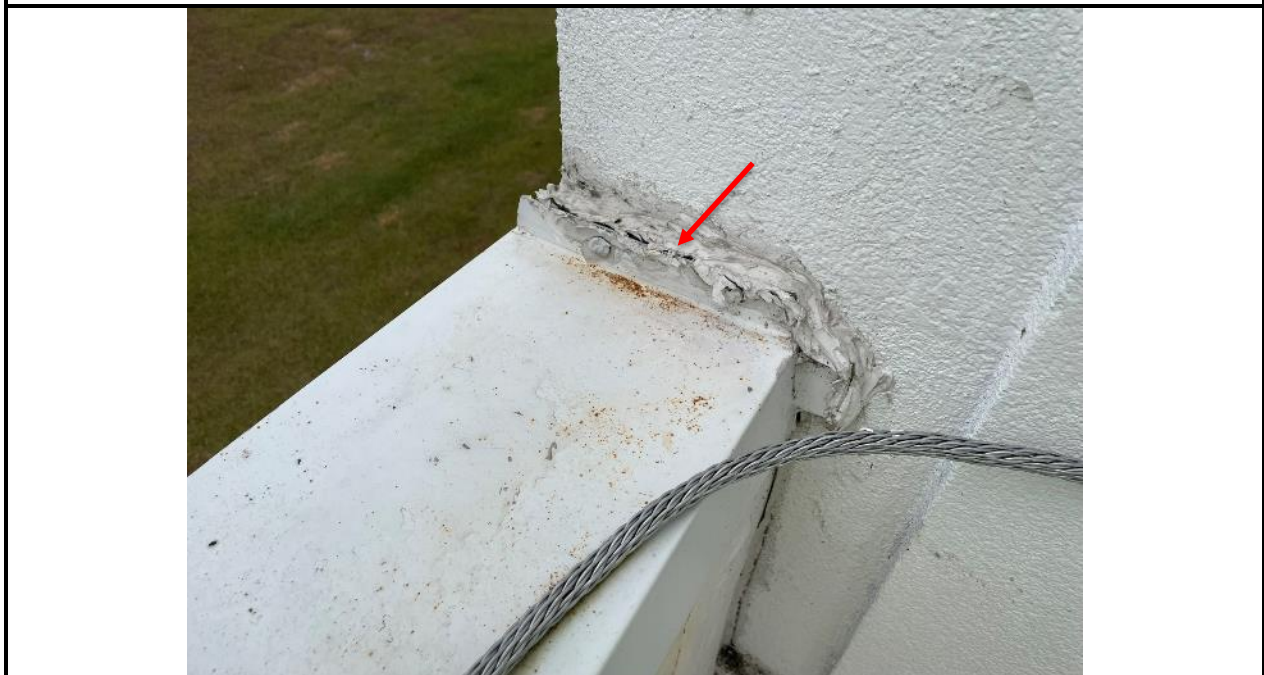
Photo 32: Deteriorated/Missing sealant along joints at building component transitions
