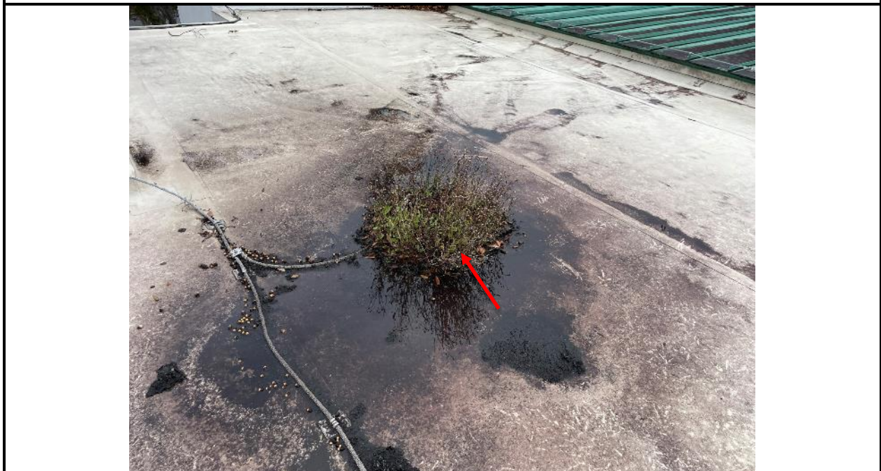
Photo 62: Vegetative debris situated on roofing membrane.
