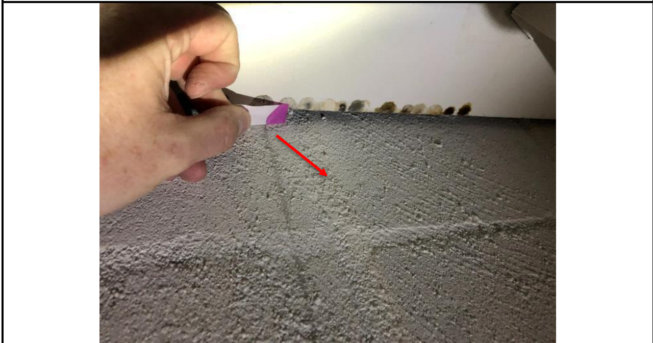
Photo 108: Test location #2 - water was visually observed and detected utilizing infrared thermography streaming down the CMU block wall at the steel girder/joist and roof deck transition as well as dripping onto the HVAC ductwork and ceiling components.
