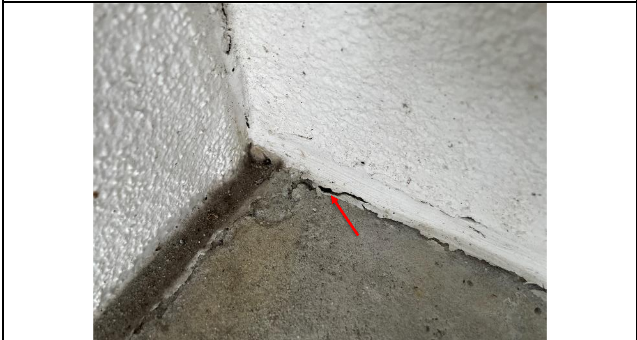
Photo 86: Deteriorated/Missing/Unadhered sealant joint details along concrete flatwork to exterior wall transitions.
