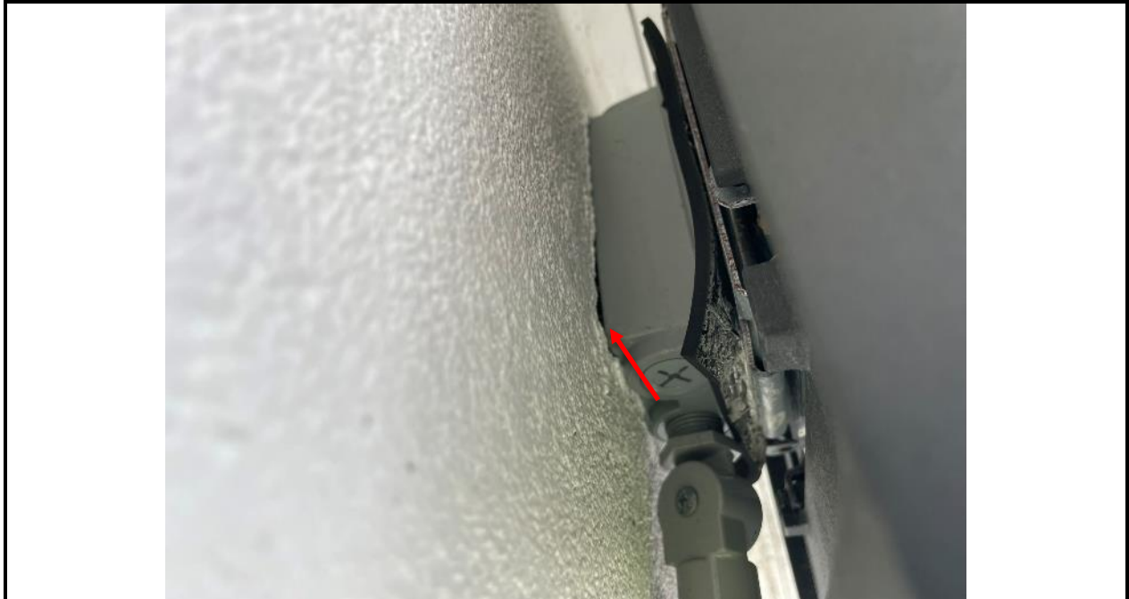
Photo 49: Unsealed through-wall penetrations.
