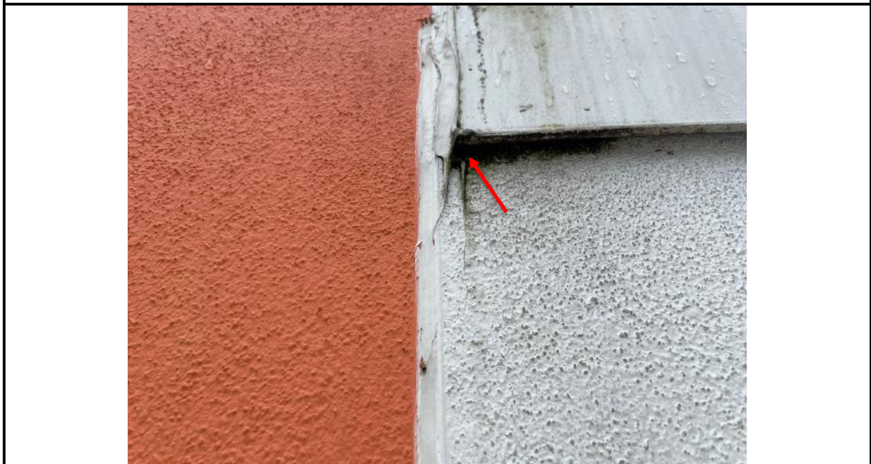
Photo 70: Separation at roof membrane transition to stucco cladding associated with elevator penthouse.
