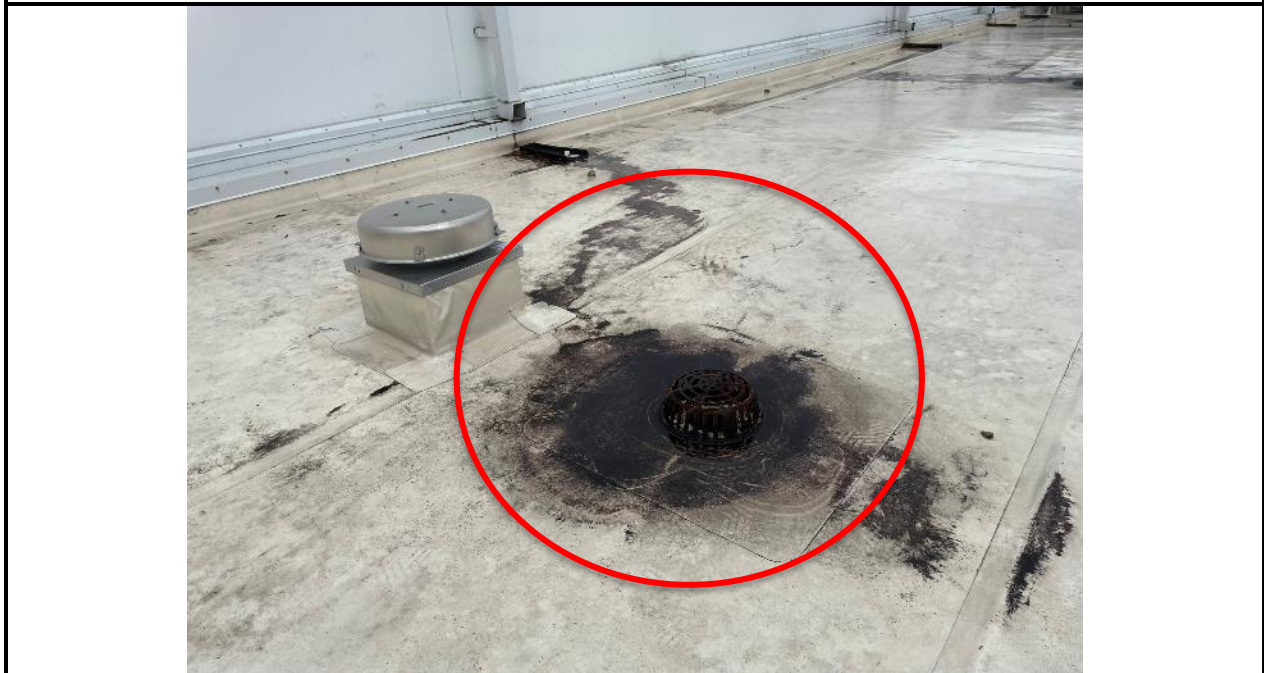
Photo 28: Stained roofing surfaces (membrane).
