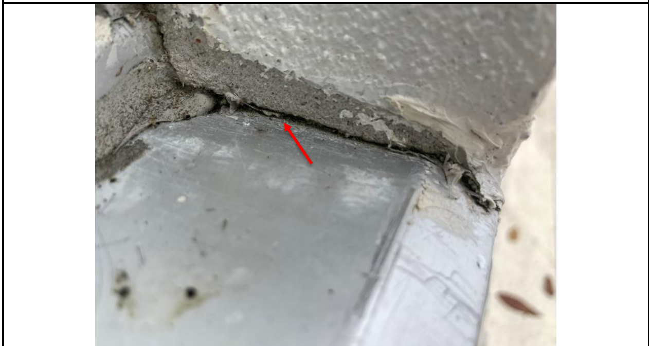
Photo 60: Openings at window assemblies' sill flashing corner transitions to adjacent construction.
