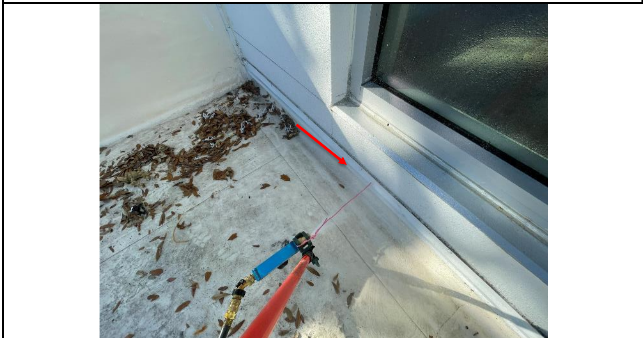
Photo 118: Test location # 6 - water was applied along the metal counter flashing transitions with sealant joints between the 1 st floor roof membrane and the adjacent construction where voids and unadhered sealant were observed beneath the window assemblies.
