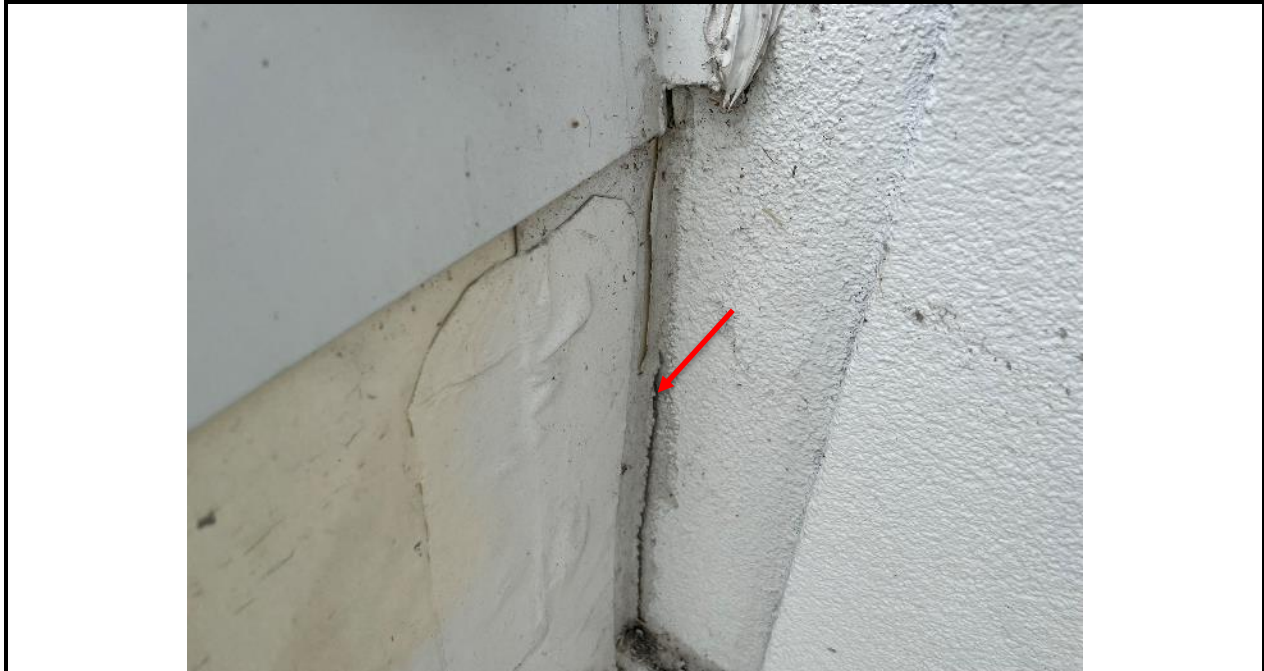
Photo 33: Deteriorated/Missing sealant along joints at building component transitions
