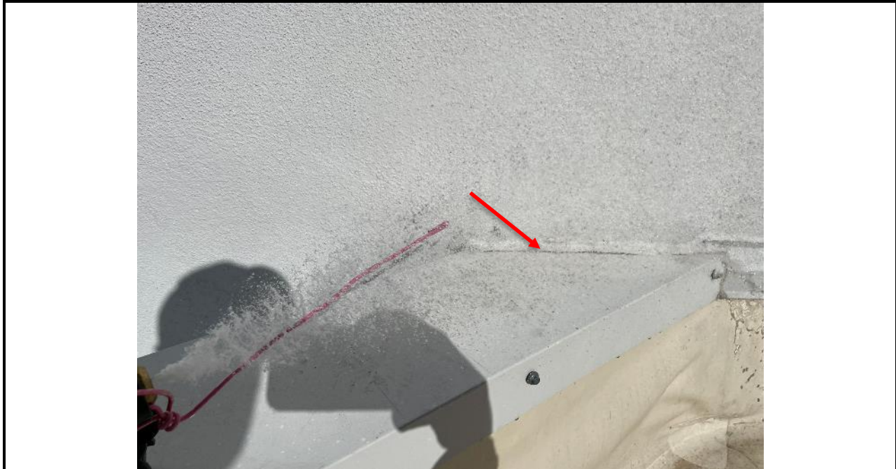
Photo 101: Test location #1 - water was applied along the roof penetrations including roof drain, deteriorated/missing sealant at roof penetrations (VTR) and building component transitions (coping cap to stucco cladding).
