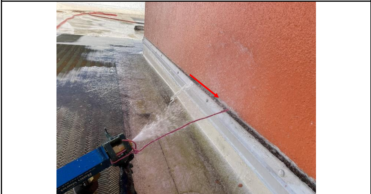
Photo 106: Test location #2 - water was applied along the metal counter flashing transition with sealant joints between the 1 st floor roof membrane and the adjacent construction (elevator shaft) where voids and unadhered sealant were observed.
