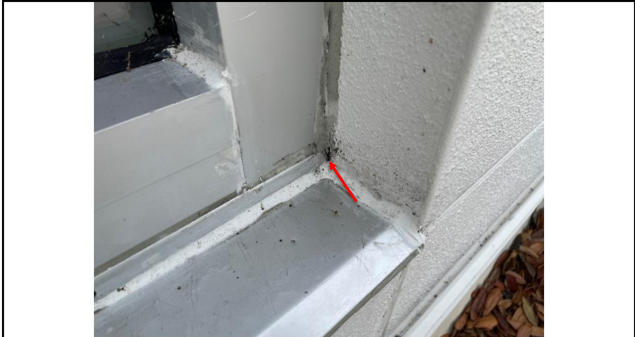
Photo 45: Void in sealant along window perimeter sealant joint transition to adjacent construction.
