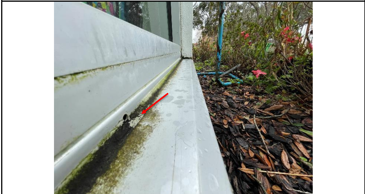
Photo 40: Sill flashing associated with window systems appears to have a negative slope back towards building exteriors creating stains and mildew growth.
