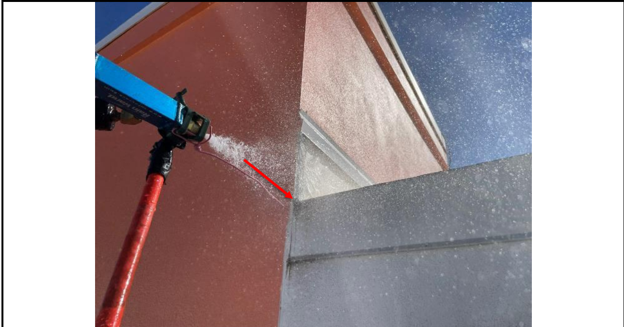
Photo 107: Test location #2 - water was applied along the observed separation at the roof membrane (covering the roof access door area) transition to the stucco cladding associated with the elevator penthouse.
