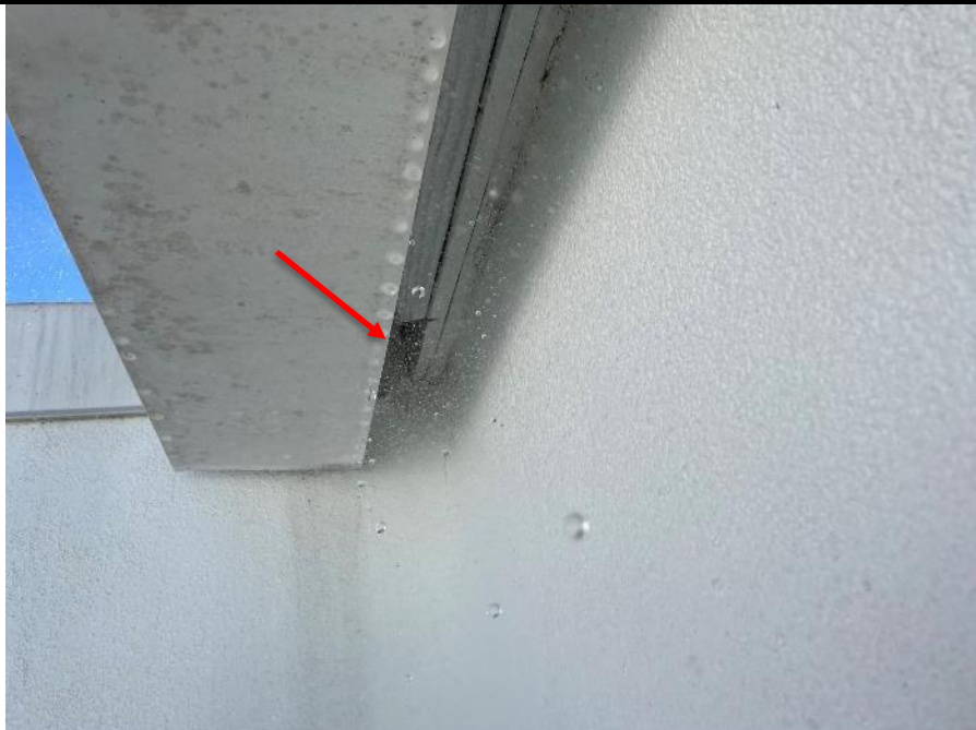
Photo 114: Test location #4 - water was applied to the observed open condition at the transition between areas of original construction (wood fascia) to new construction (stucco cladding) behind the gutter system.
