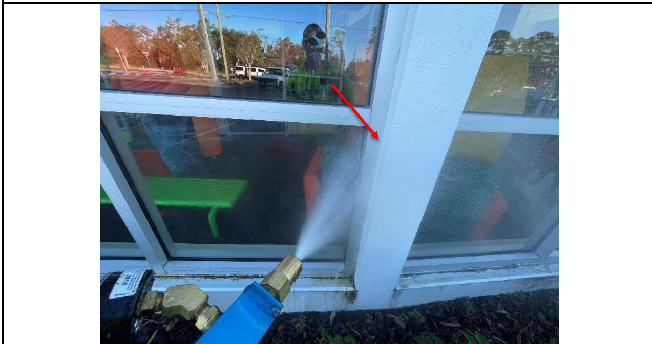
Photo 126: Test Location #7 – water along three (3) of the storefront window assemblies including voids beneath the sill flashing, voids in the perimeter sealant joints, openings at the lower corners, and negative sloped sill flashing detail associated with the fixed window assemblies.
