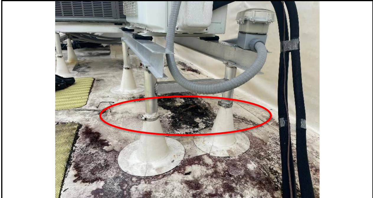
Photo 37: Deteriorated/Missing sealant at roof penetration transitions.
