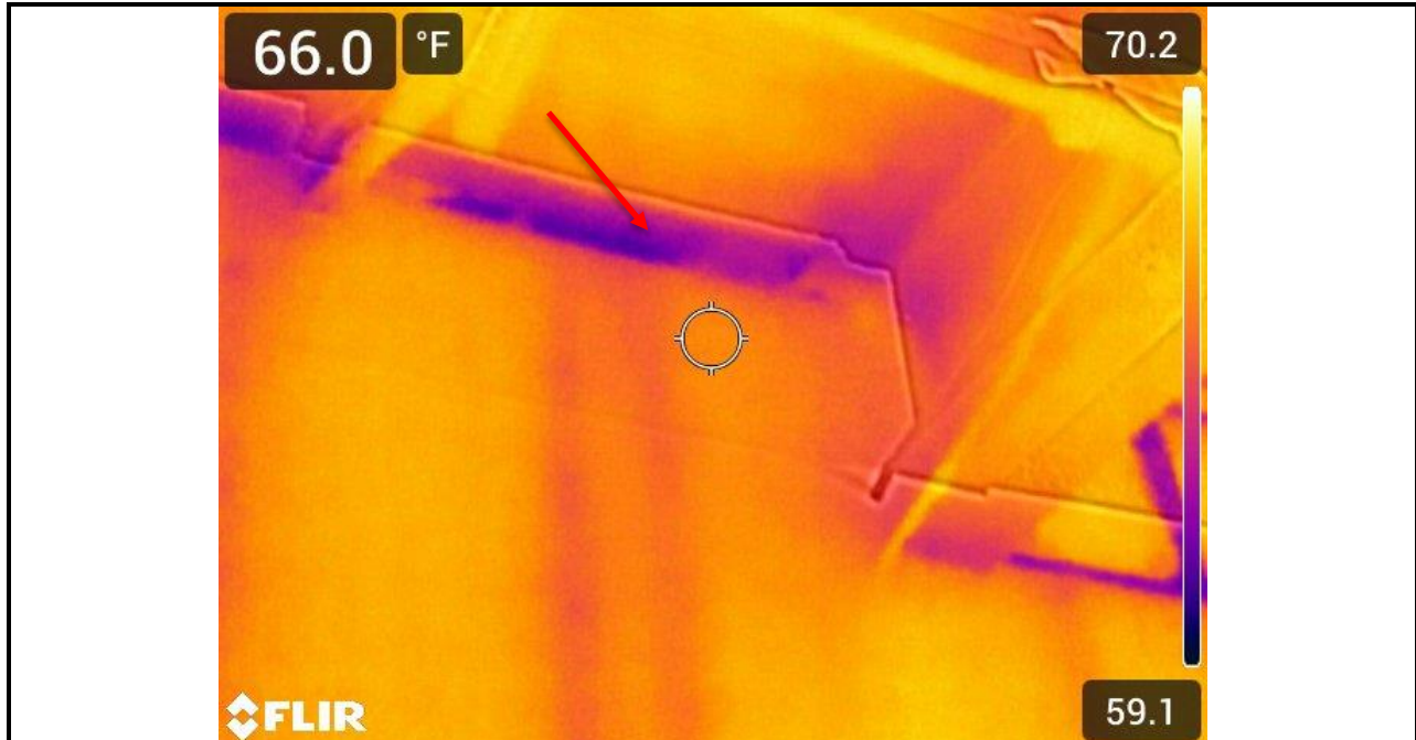
Photo 123: Test Location #6 - Temperature variances indicative of suspected surface and subsurface moisture trapped within the interior construction components were detected utilizing infrared thermography.
