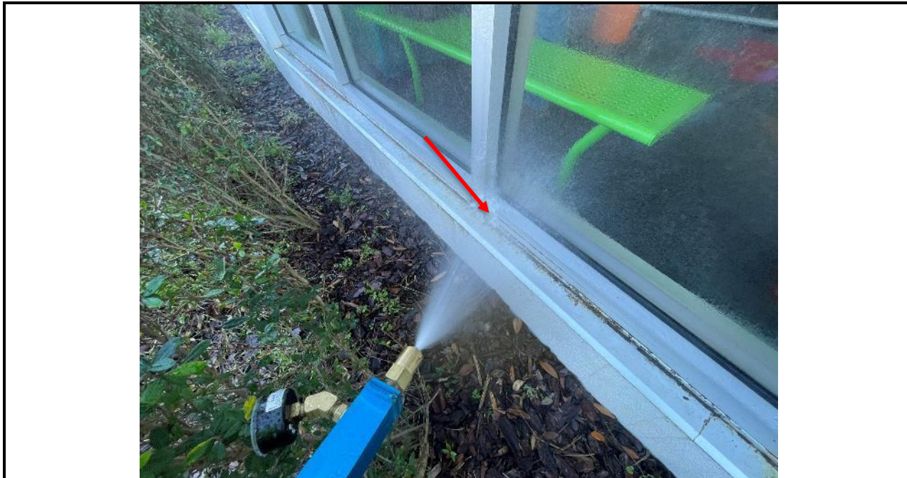
Photo 125: Test Location #7 – water along three (3) of the storefront window assemblies including voids beneath the sill flashing, voids in the perimeter sealant joints, openings at the lower corners, and negative sloped sill flashing detail associated with the fixed window assemblies.
