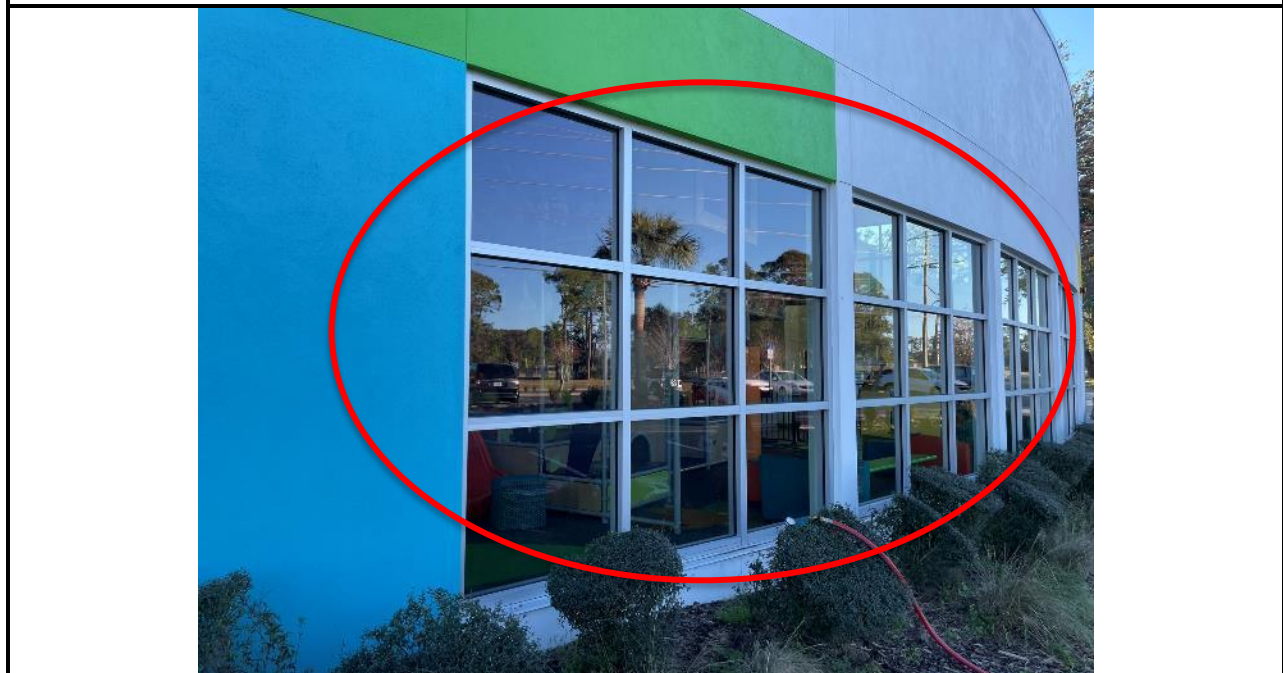
Photo 124: Test Location #7 – water along three (3) of the storefront window assemblies including voids beneath the sill flashing, voids in the perimeter sealant joints, openings at the lower corners, and negative sloped sill flashing detail associated with the fixed window assemblies.
