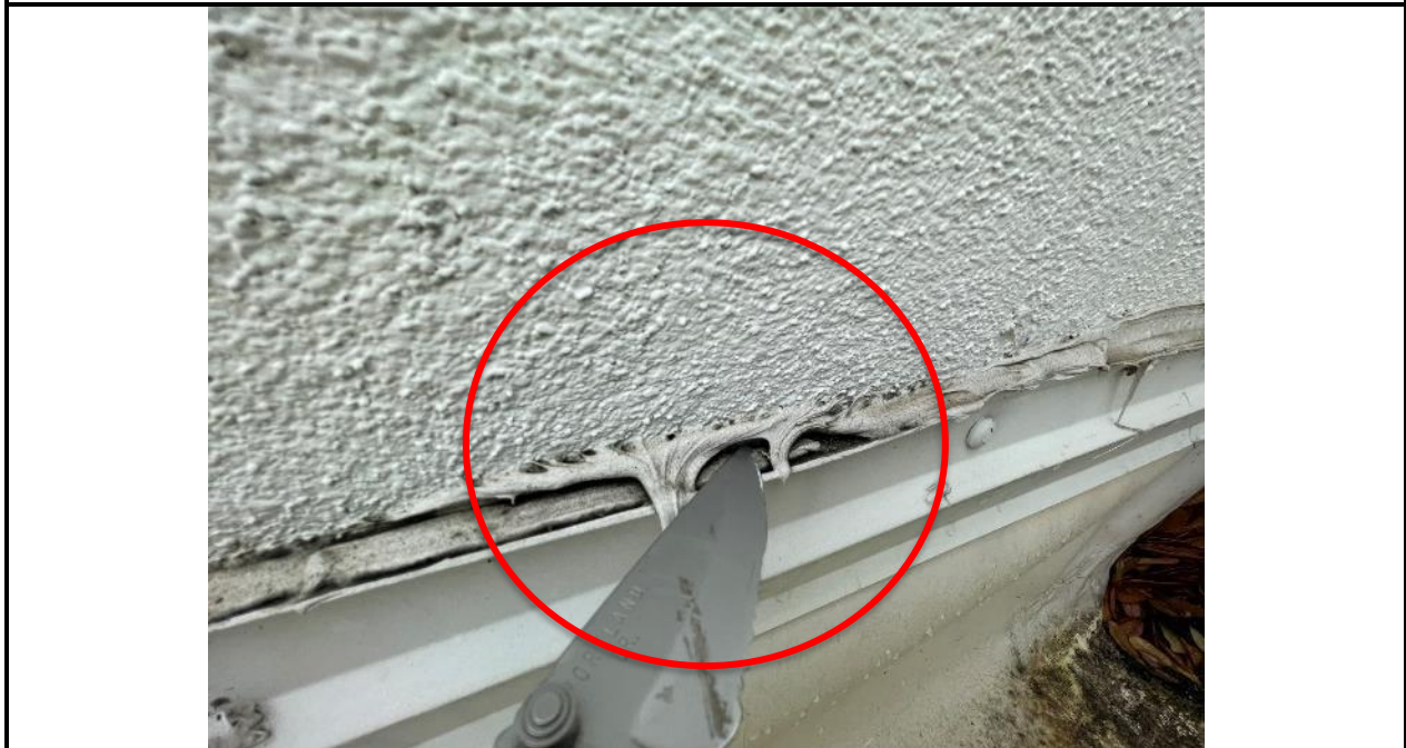
Photo 30: Deteriorated/Missing sealant along joints at building component transitions
