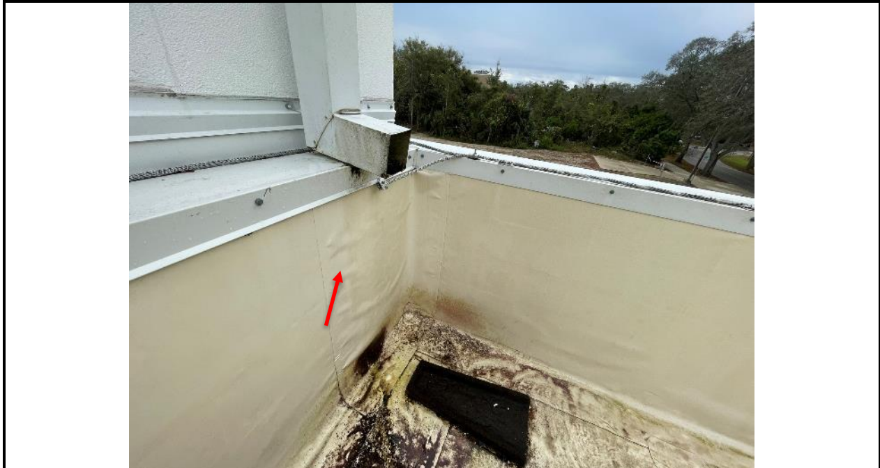
Photo 65: Blisters/Wrinkles in adhered membrane associated with parapet walls.
