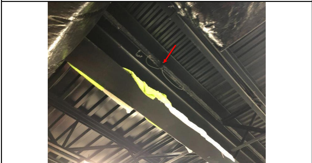
Photo 92: Evidence of previous moisture infiltration including stained interior ceiling components, stained/efflorescence on joists and metal decking, voids in the interior perimeter sealant between window and drywall, and water stains on interior faces of storefront window framing members.
