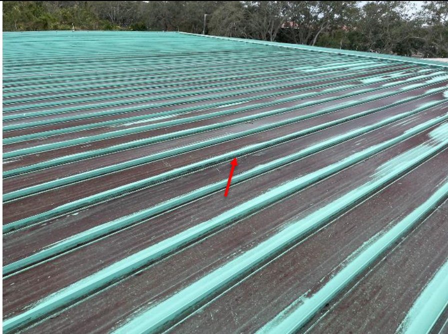
Photo 81: Stained metal panels associated with standing seam roof system.
