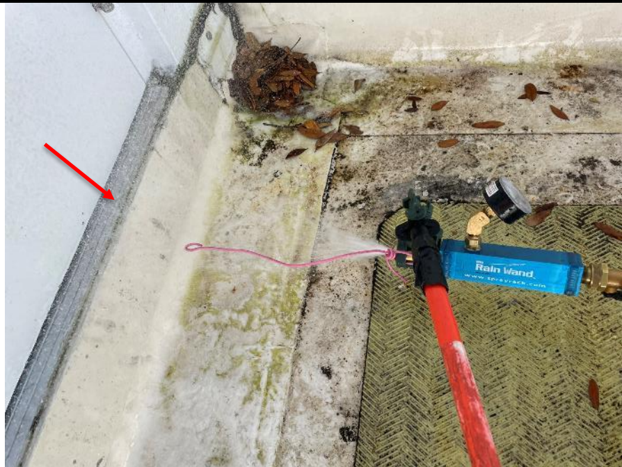
Photo 110: Test location #3 -water was applied along the metal counter flashing transitions with sealant joints beneath the roof access door where voids and unadhered sealant were observed.
