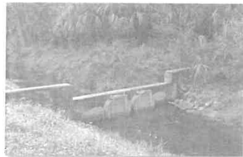
Sanders Road outfall ditch control structure (downstream view).
