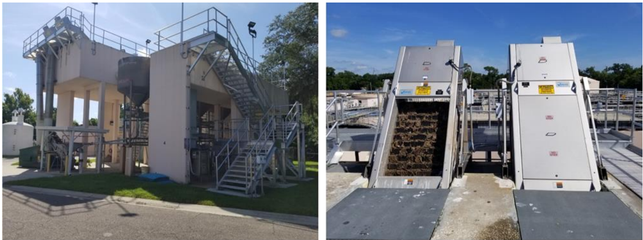
FIGURE 34: EXISTING HEADWORKS AND BARSCREENS
