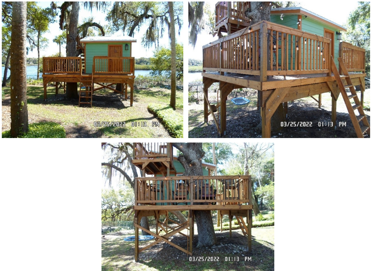
Pictures taken of the elevated accessory structure by Code Enforcement in March 2022
