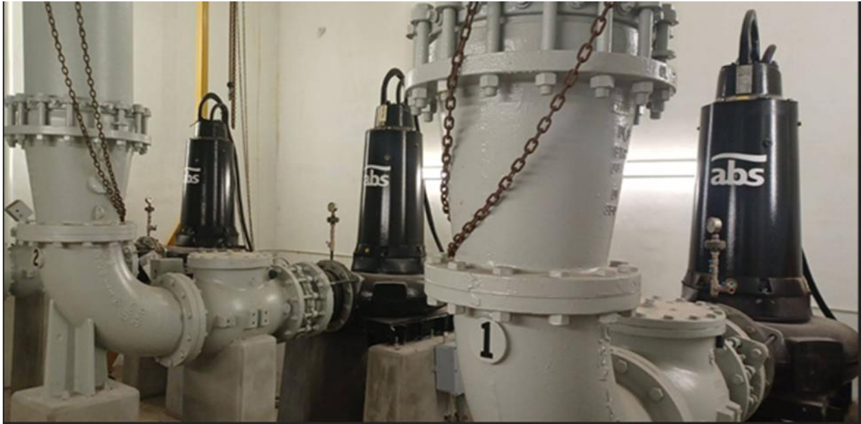
FIGURE 25: DRY PIT SUBMERSIBLE PUMPS
