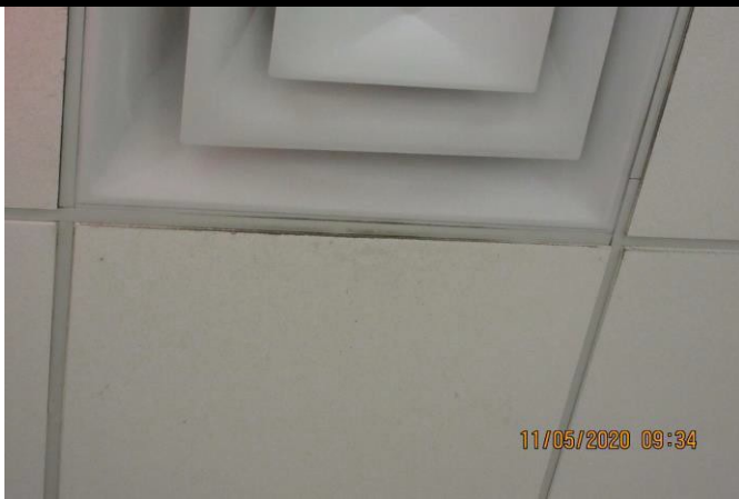
Photograph 13 1st Floor East Corridor – Minor Dust on Ceiling Tile
