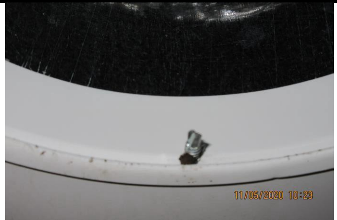
Photograph 46 Captain Fisher's Office Discoloration on HVAC Vent
