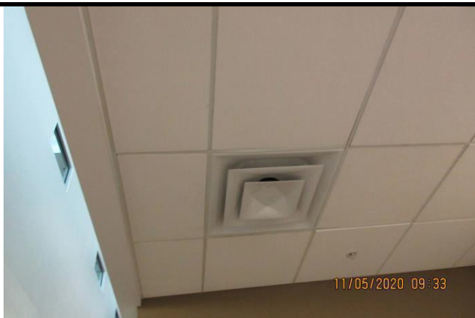
Photograph 9 1st Floor East Corridor – HVAC Vent
