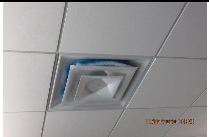
Photograph 22 Room 227 - Filter added above HVAC Vent
