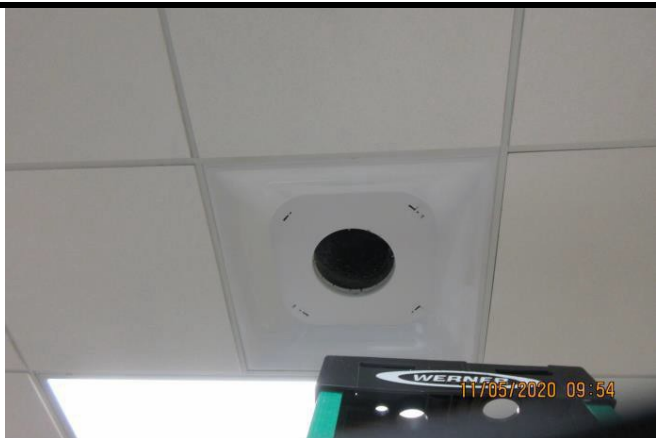
Photograph 31 Room 227 - HVAC Duct
