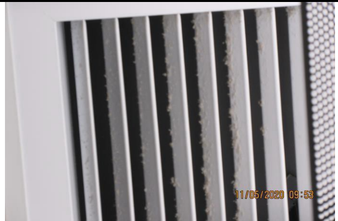
Photograph 20 Room 227 - Dust and Debris on HVAC Return
