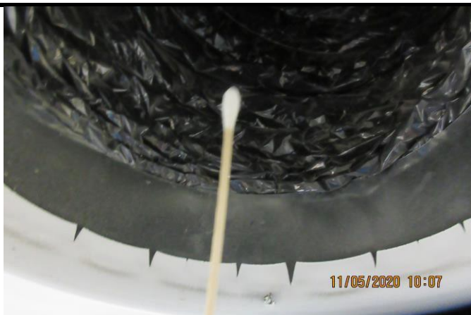
Photograph 35 Room 227 - Discoloration inside HVAC Duct
