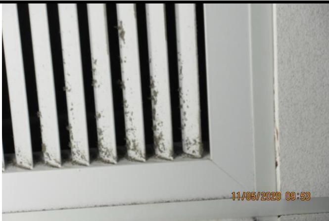
Photograph 21 Room 227 - Dust and Debris on HVAC Return
