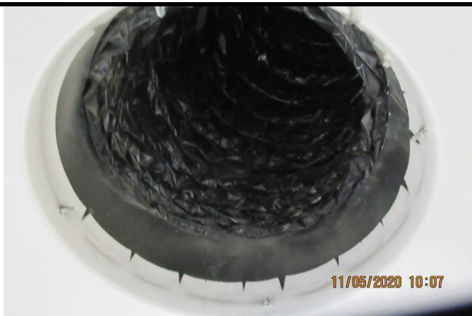
Photograph 33 Room 227 - Discoloration inside HVAC Duct
