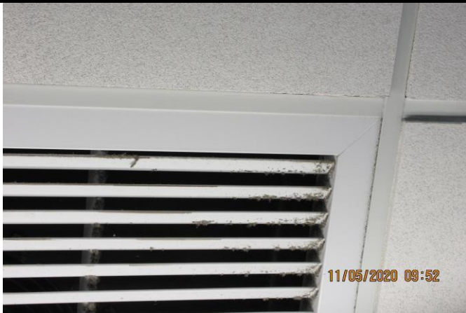
Photograph 19 Room 227 - Dust and Debris on HVAC Return
