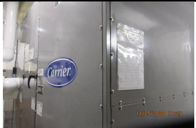
Photograph 52 Room 252 Mechanical – Carrier HVAC
