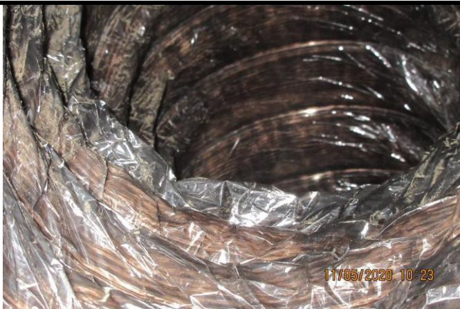
Photograph 47 Captain Fisher's Office Discoloration inside HVAC Duct
