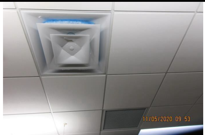
Photograph 26 Room 227 - Filter added above HVAC Vent
