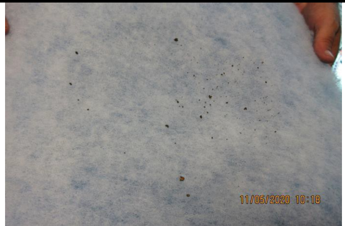
Photograph 40 Captain Fisher's Office - Black Specks on the Back of Filter
