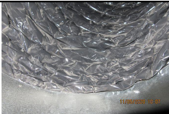
Photograph 34 Room 227 - Discoloration inside HVAC Duct
