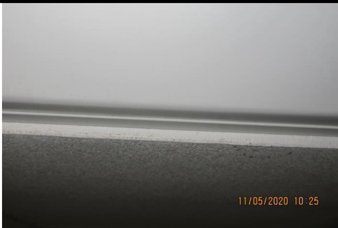
Photograph 49 Captain Fisher's Office Discoloration on Ceiling Tile by HVAC Vent
