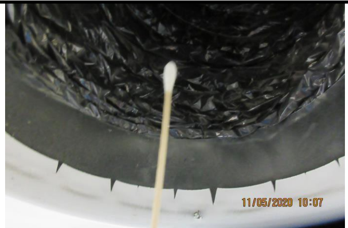
Photograph 58 Swab – Room 227 HVAC Duct
