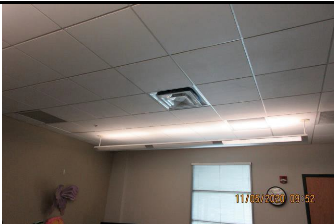
Photograph 17 Room 227 – Ceiling Tiles
