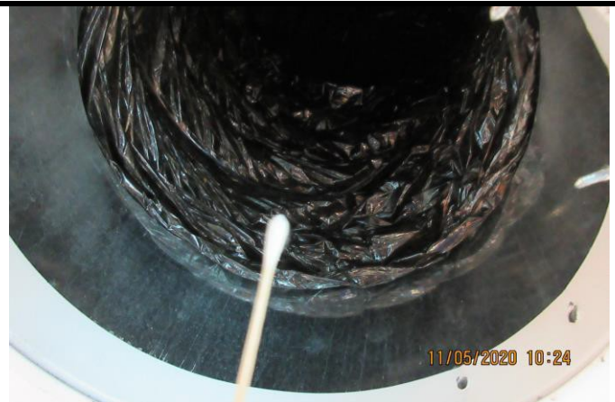
Photograph 48 Captain Fisher's Office Discoloration inside HVAC Duct
