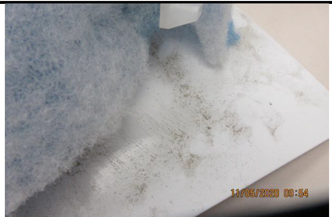
Photograph 30 Room 227 - Discoloration on the back of HVAC Vent at the Filter
