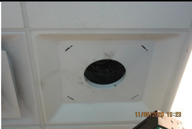
Photograph 45 Captain Fisher's Office Discoloration on HVAC Vent
