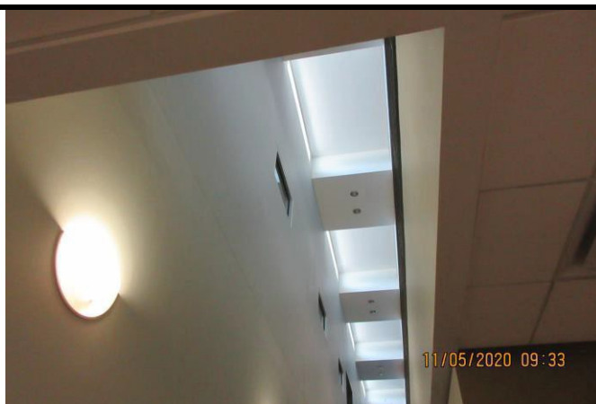
Photograph 8 1st Floor East Corridor – Open Ceiling
