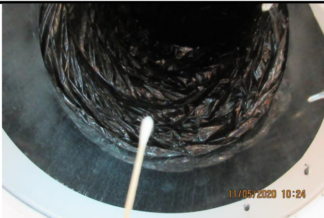
Photograph 59 Swab – Captain Fisher’s Office HVAC Duct
