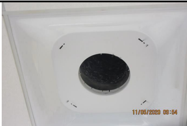
Photograph 32 Room 227 - HVAC Duct
