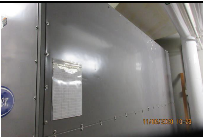
Photograph 53 Room 252 Mechanical – Carrier HVAC
