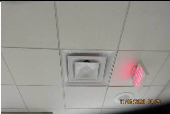
Photograph 5 1st Floor East Corridor – HVAC Vent
