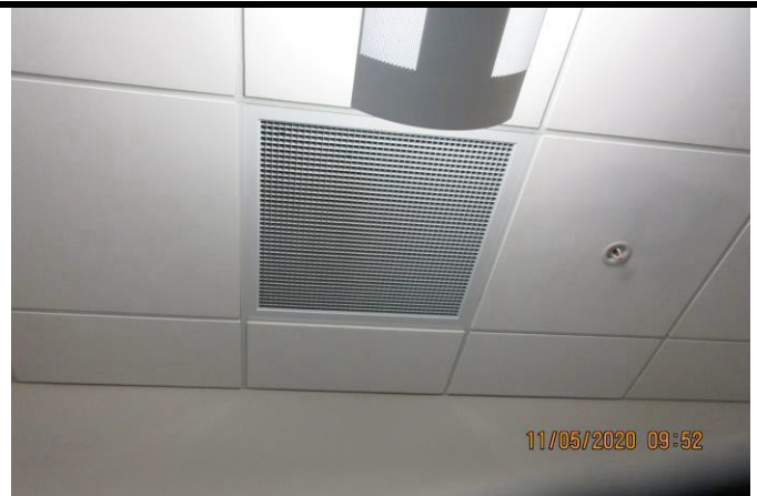
Photograph 18 Room 227 – HVAC Damper
