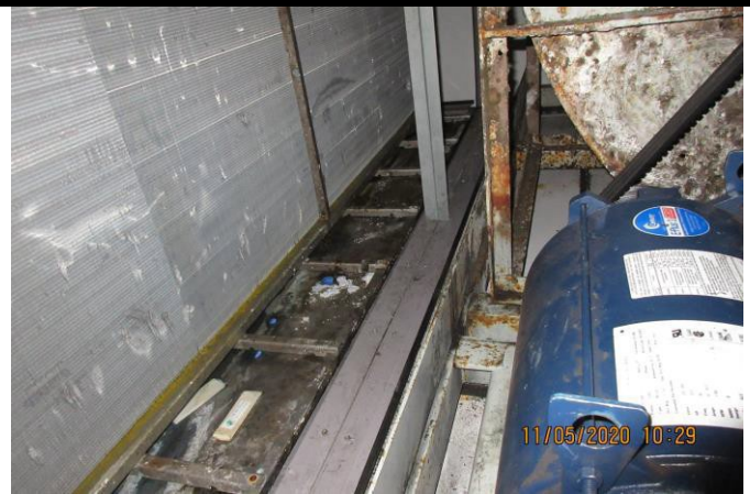
Photograph 56 Room 252 Mechanical – HVAC Coils
