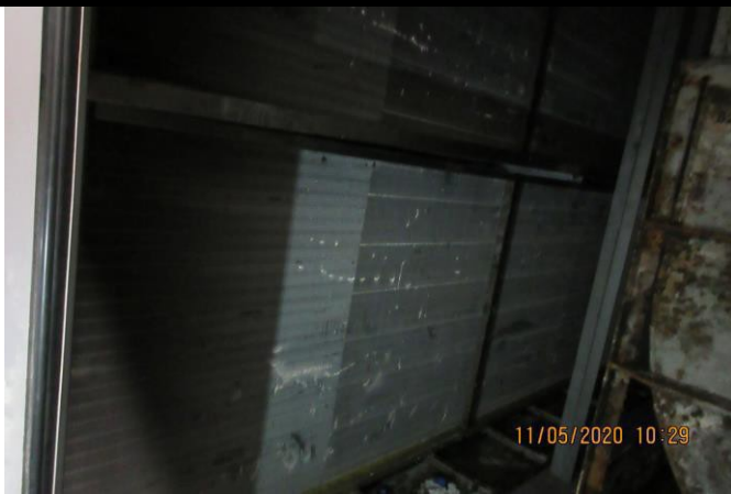
Photograph 55 Room 252 Mechanical – HVAC Coils
