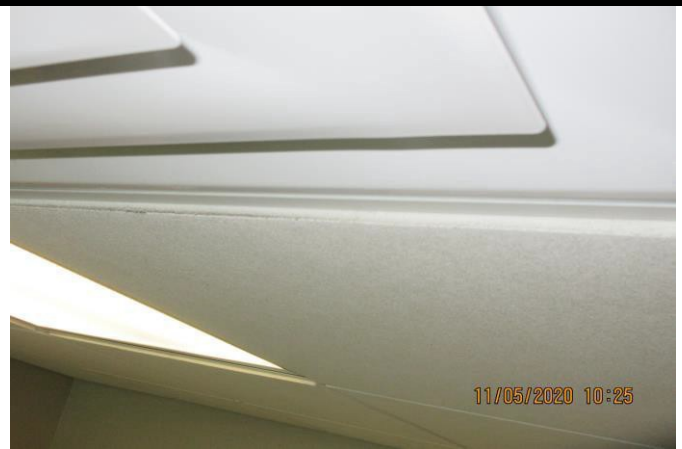
Photograph 50 Captain Fisher's Office Discoloration on Ceiling Tile by HVAC Vent
