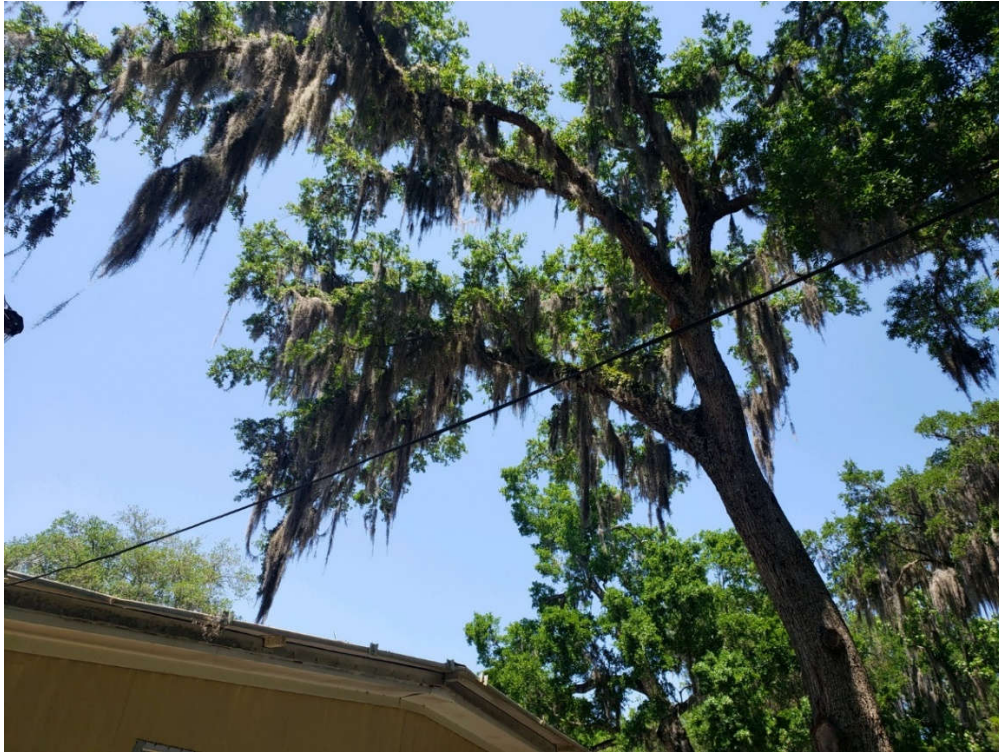
Figure 4 - Photo of the tree canopy overhanging the roof.
