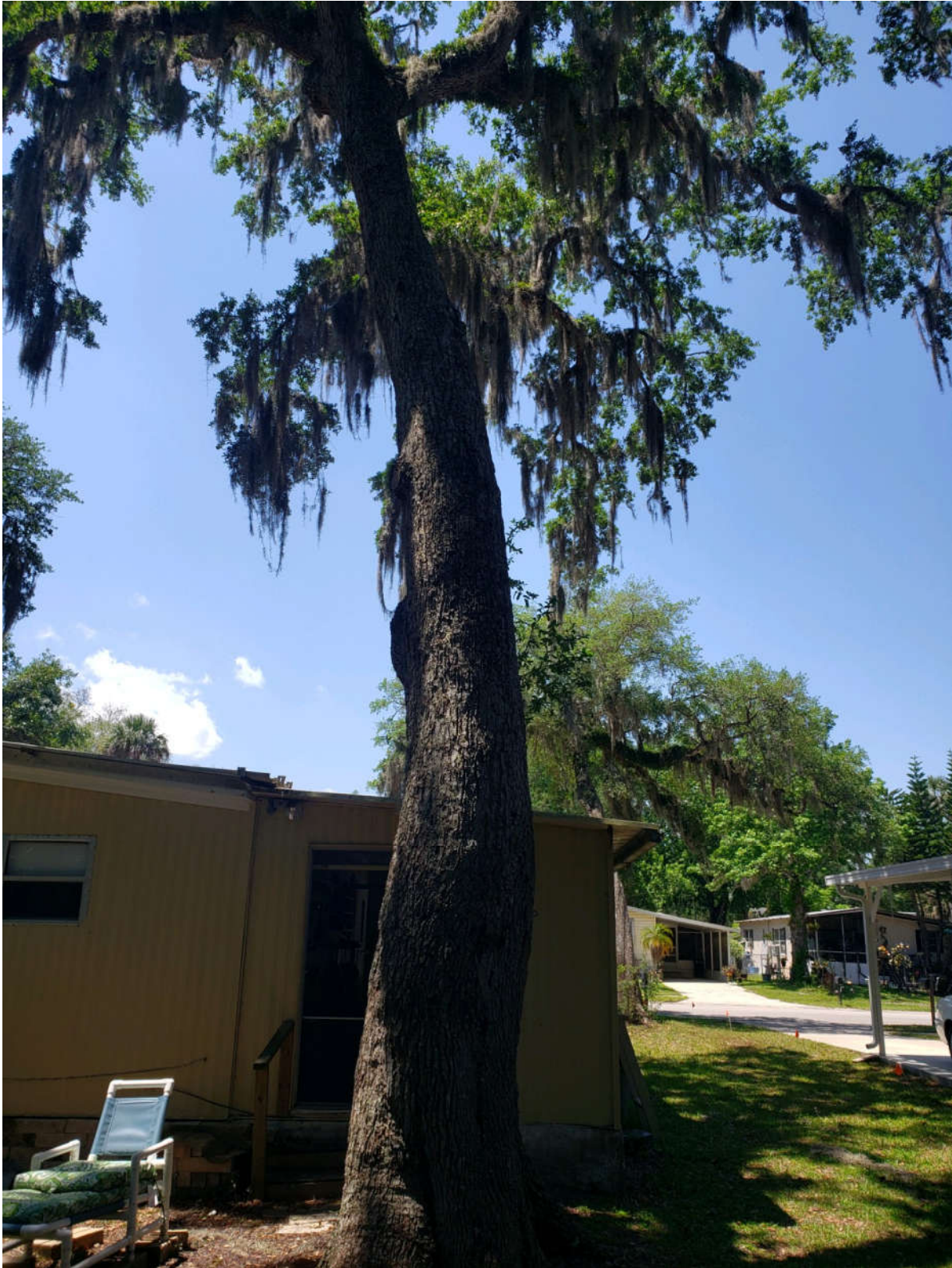
Figure 2- Photo of the tree taken from the rear of the property showing the tree trunk curving towards the home and the tree canopy overhanging the roof in the background.
