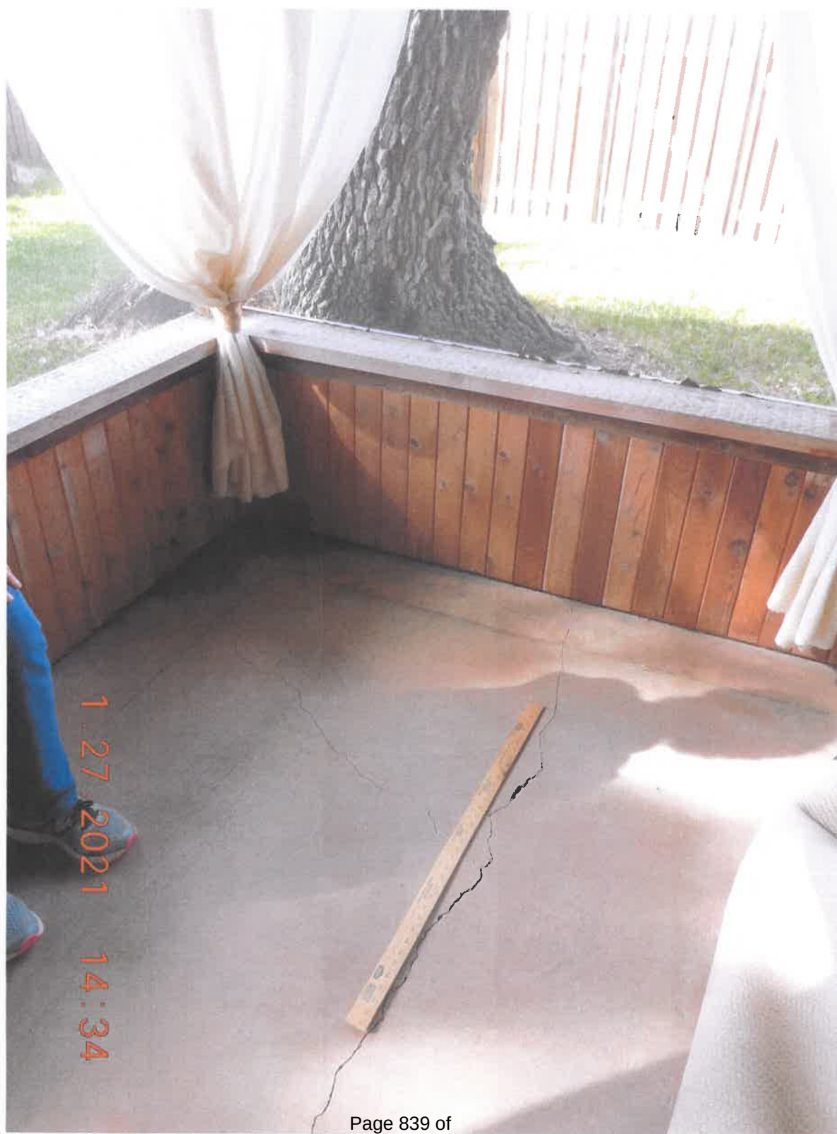
Photo taken inside the enclosed porch that shows a portion of the crack in the foundation
