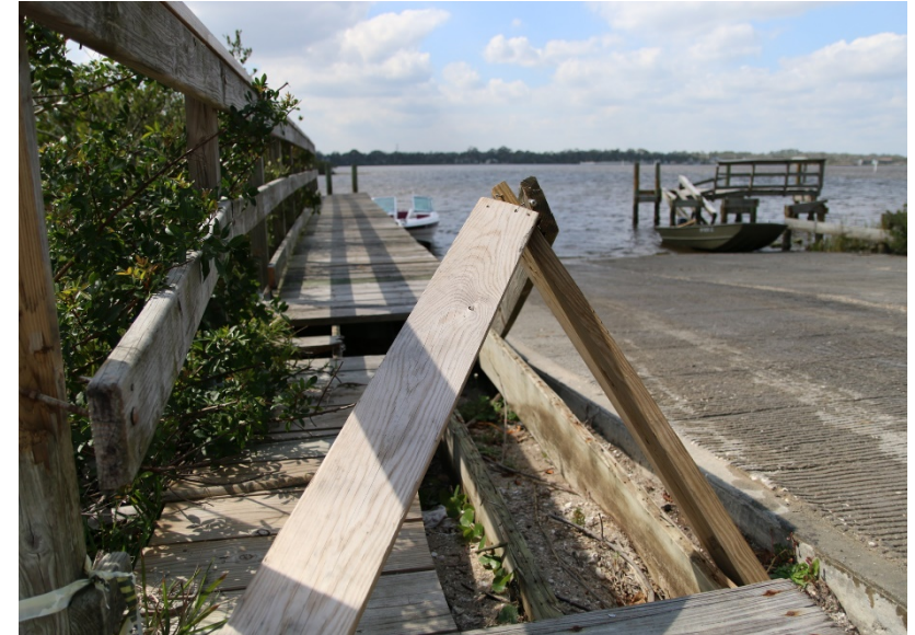
Hurricane Damage at Causeway Park
